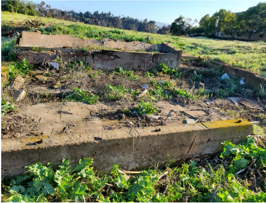
Photograph #9 Concrete foundation debris in the central-eastern portion of the Site.
