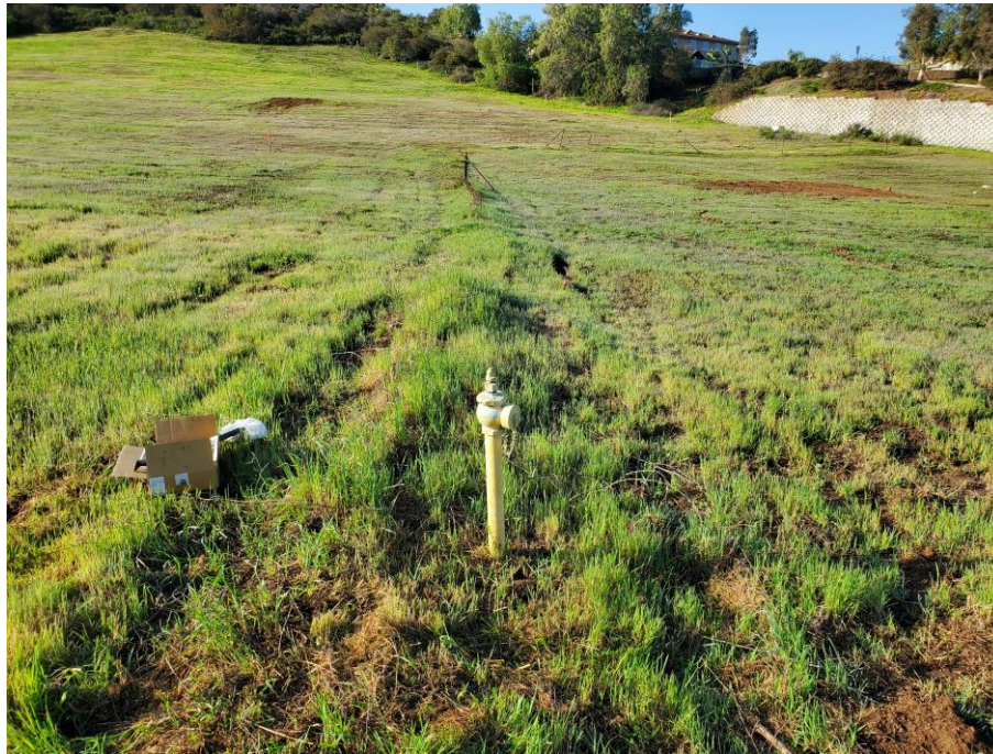
Photograph #11 Water line located in the central-northern portion of the Site.
