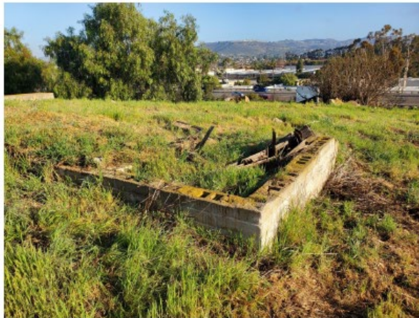
Photograph #8 Concrete foundation debris in central-eastern portion of the Site.
