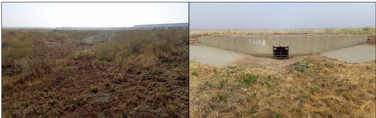
Figure 11. Earthen drainage channel in the APE (Site 33-024853). Left : overview to the southeast; right : culvert under Taxiway A (Feature 1), view to the northwest. (Photographs taken on June 23, 2020)
