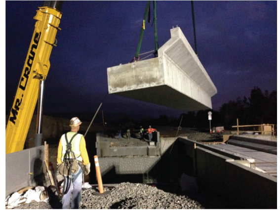
Overhead protection is required when moving heavy objects over Metro ROW or in areas designated for public use.
