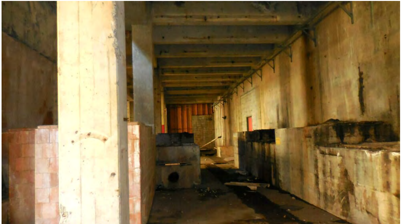
Figure 54. Interior of Machine Building – large amounts of light and airflow, not conducive to bat roosting activity, even in more protected locations such as this concrete wall and girder ceiling area.
