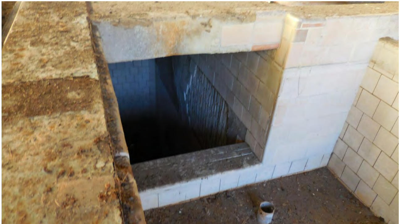
Figure 56. Enclosed and partially-enclosed rooms inside Machine Building – no signs of past or present use by bats.
