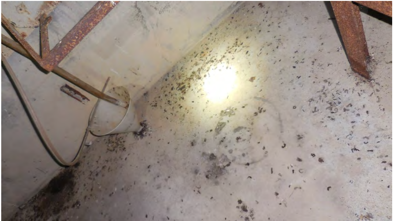
Figure 13. Bat fecal pellets observed in Filter/Softener Building. Some rodent activity also noted.
