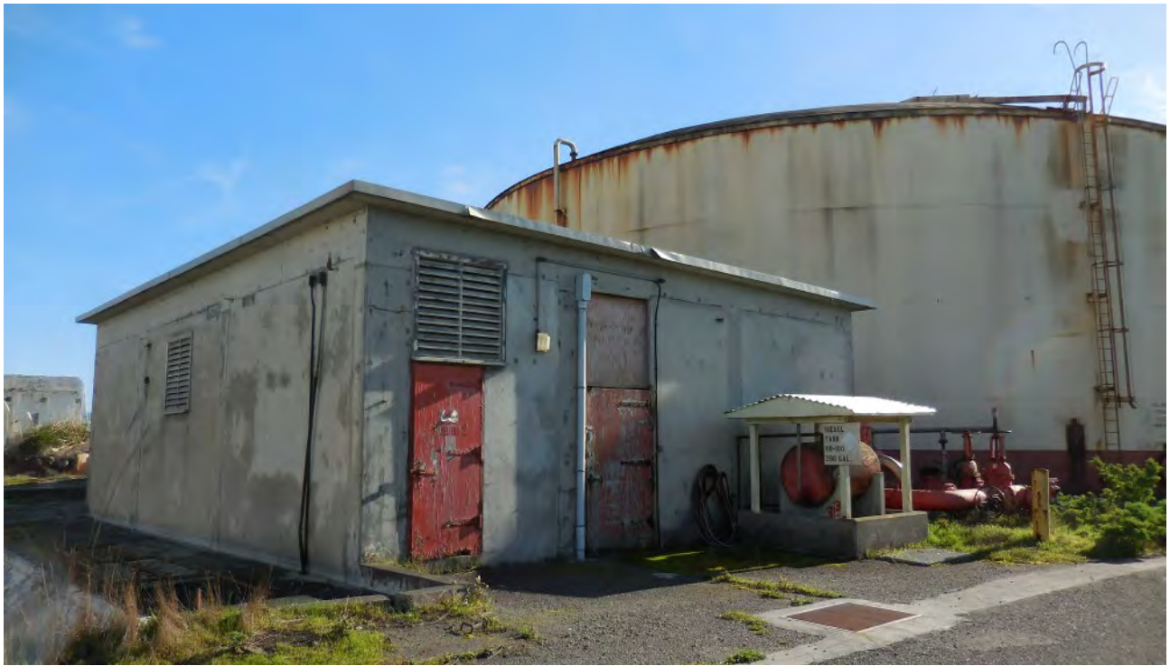
Figure 3. Pump House. Bat activity noted throughout. Remove only during seasonal periods of bat activity after conducting partial dismantling/deterrence measures as detailed in text.
