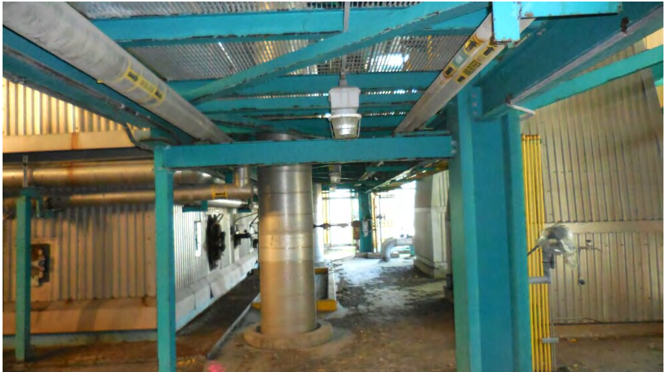
Figure 20. Interior of 12-Story Boiler Building. Large amounts of light and in some locations, airflow, not conducive to bat roosting activity. No signs of past or present use found.
