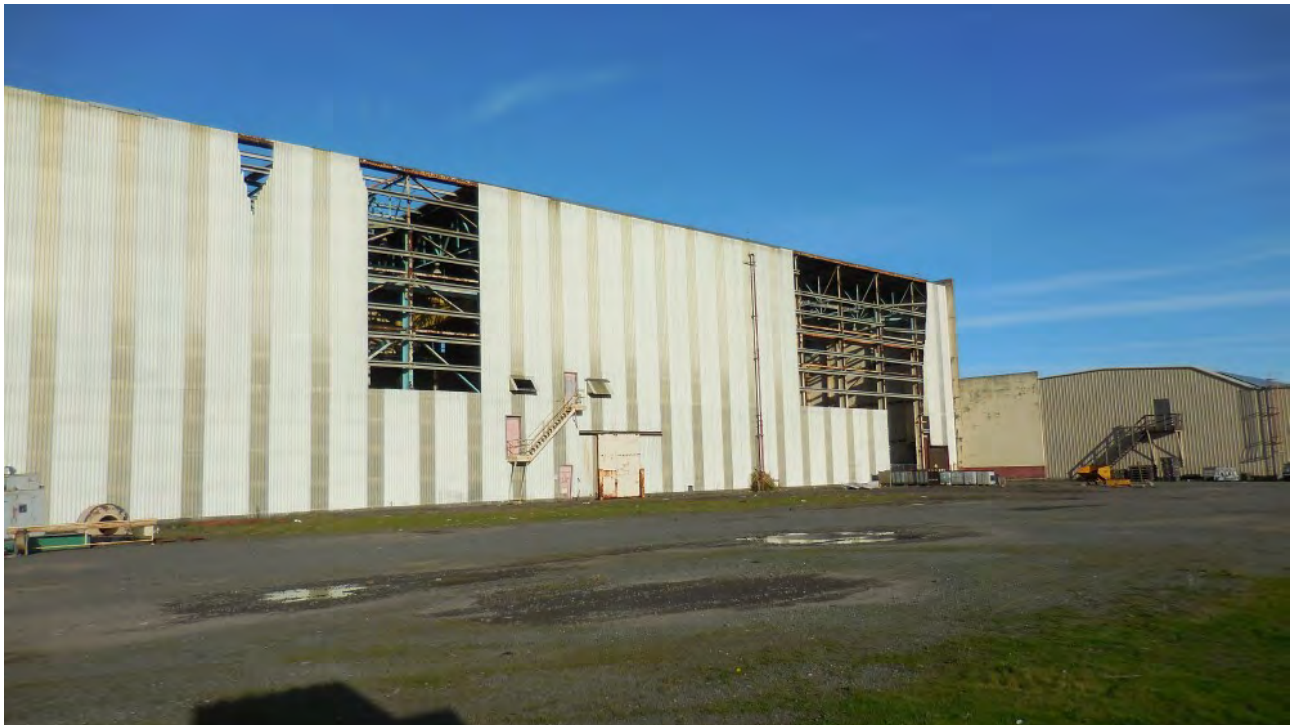
Figure 50. Machine Building. Extremely large structure has many large openings in walls and roof. No signs of past or present use by bats observed around exterior, or in interior large open spaces or enclosed rooms.
