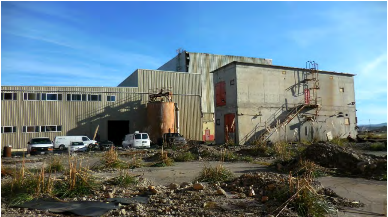
Figure 42. Existing Offices at left, Silo (tank), Warehouse and Shared Spaces in middle portion of large structure, and Structure (2-story, concrete) in foreground at right. No signs of past or present use by bats in any of these structures.
