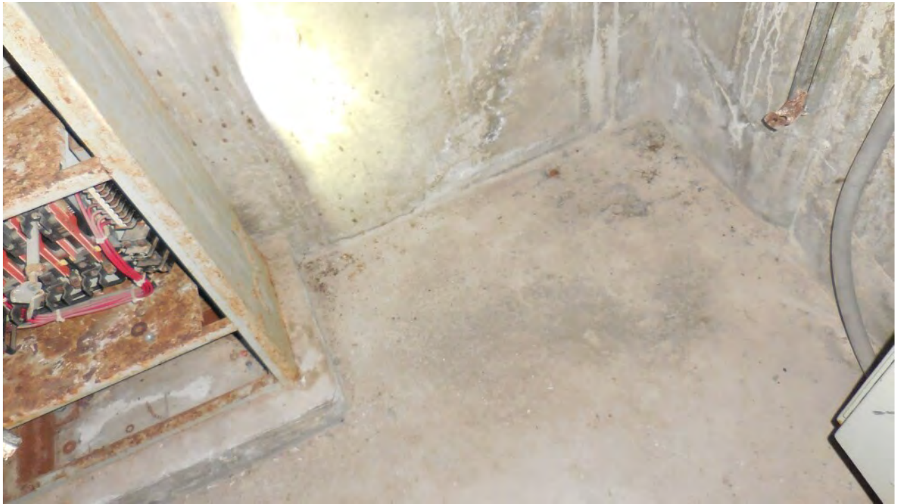
Figure 9. Building SUB FL.2. Bat activity noted in several interior locations.
