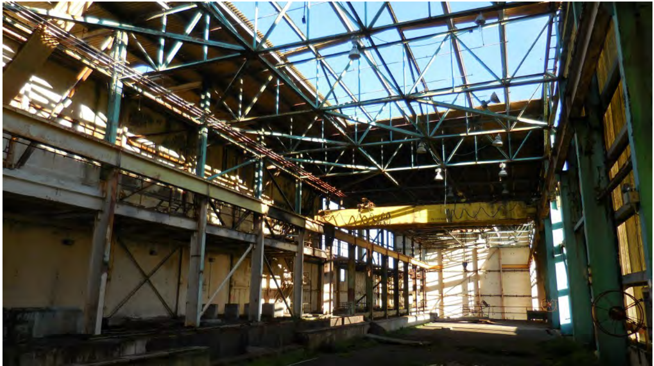
Figure 52. Interior of Machine Building – large amounts of light and airflow, not conducive to bat roosting activity.
