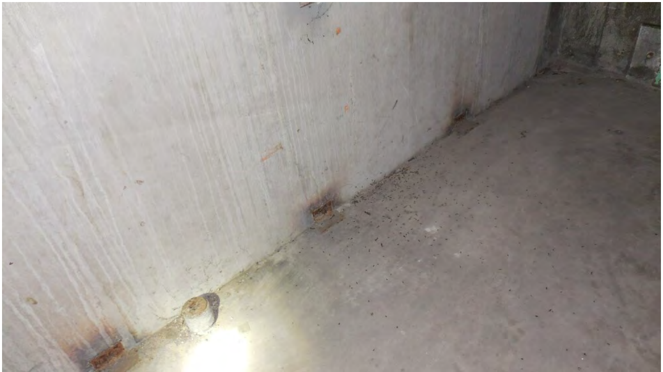
Figure 6. Bat fecal pellets noted in several locations throughout Pump House.
