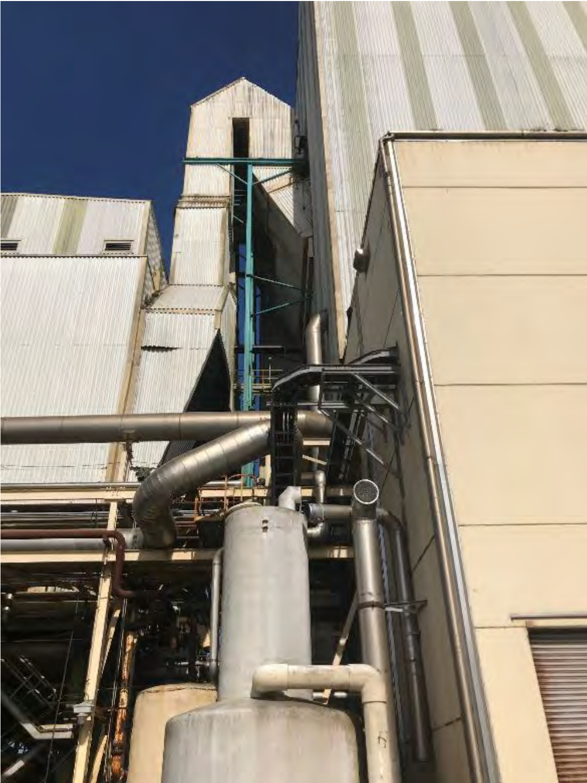
Photo 14. Closer view of main boiler building with inactive nest visible (unknown species, likely Common Raven).
