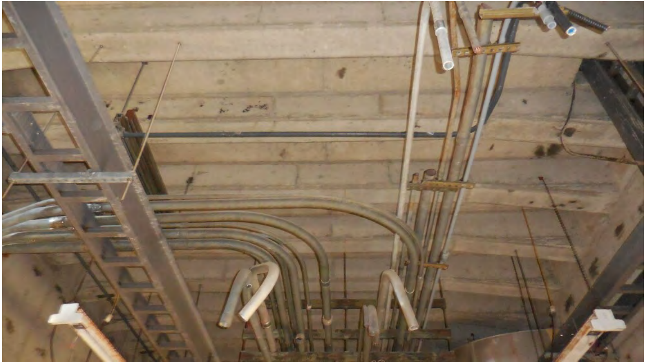
Figure 49. T-beam ceiling girders provide good suitable habitat for bats, although no signs of use were present. However, Structure and Structure 2, identical in construction, should be removed prior to removal of bat-occupied structures to prevent bats abandoning those buildings from moving into these structures.
