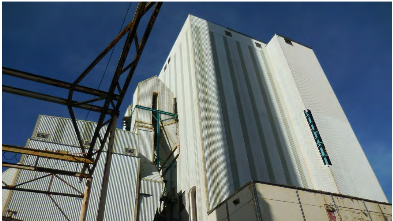
Figure 16. East-facing portion of 12-Story Boiler Building and attached structure. No signs of past or present use by bats.
