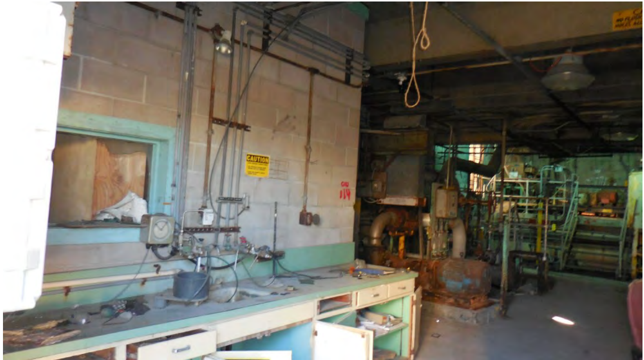
Figure 12. Interior of Filter/Softener Tank Building. Evidence of use by bats inside this structure, but not present in the attached, J-shaped Tank Support Building.
