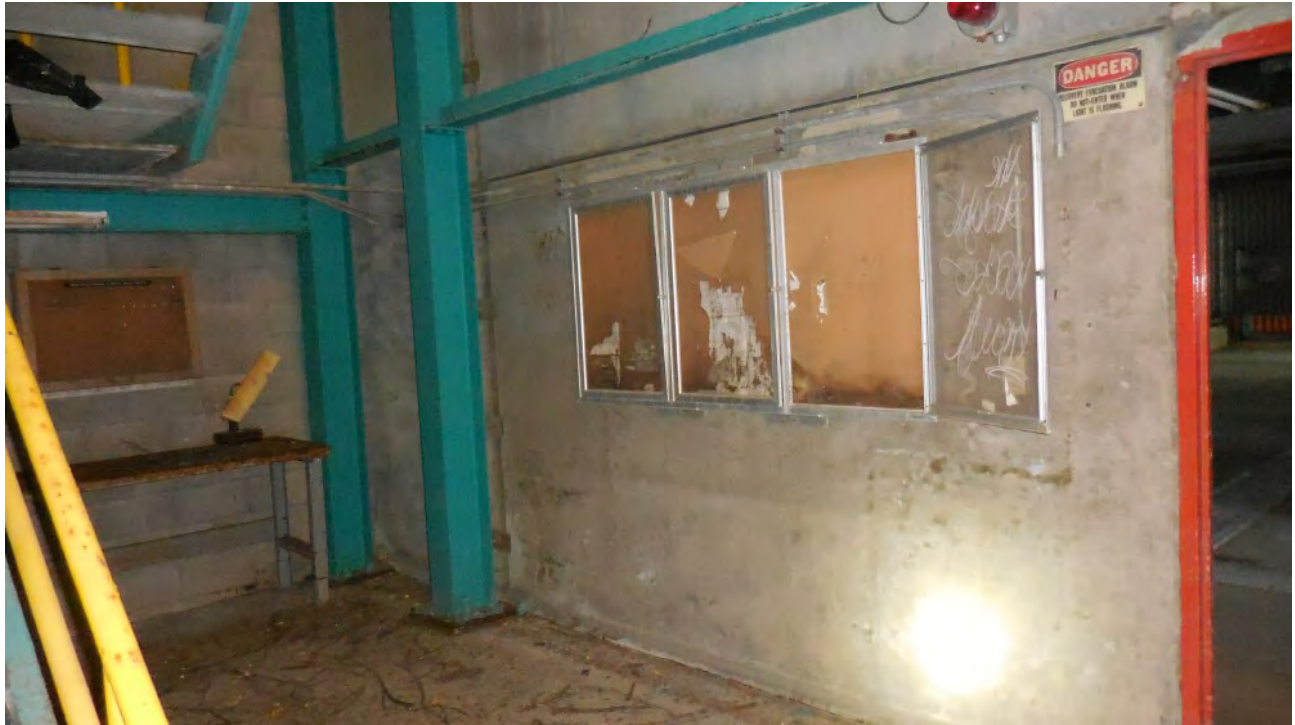
Figure 19. Interior of 12-Story Boiler Building. Large amounts of light and in some locations, airflow, not conducive to bat roosting activity. No signs of past or present use found.
