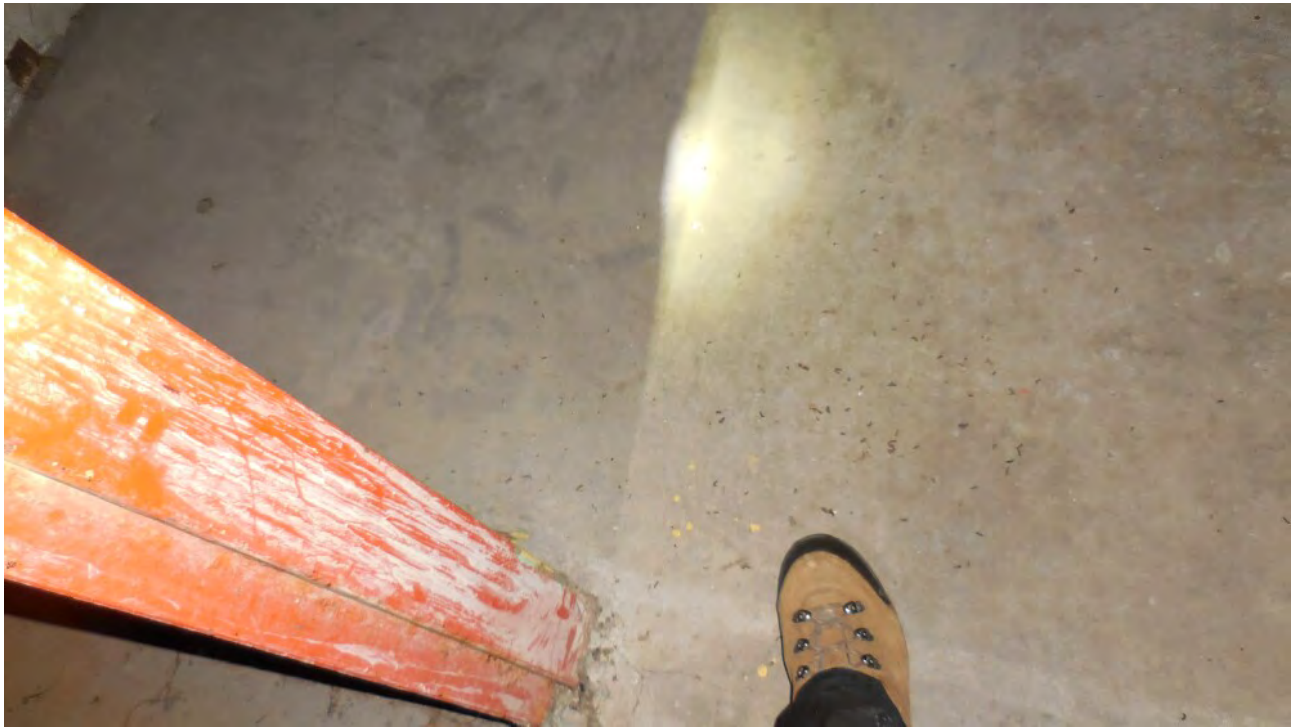
Figure 5. Bat fecal pellets noted in several locations throughout Pump House.
