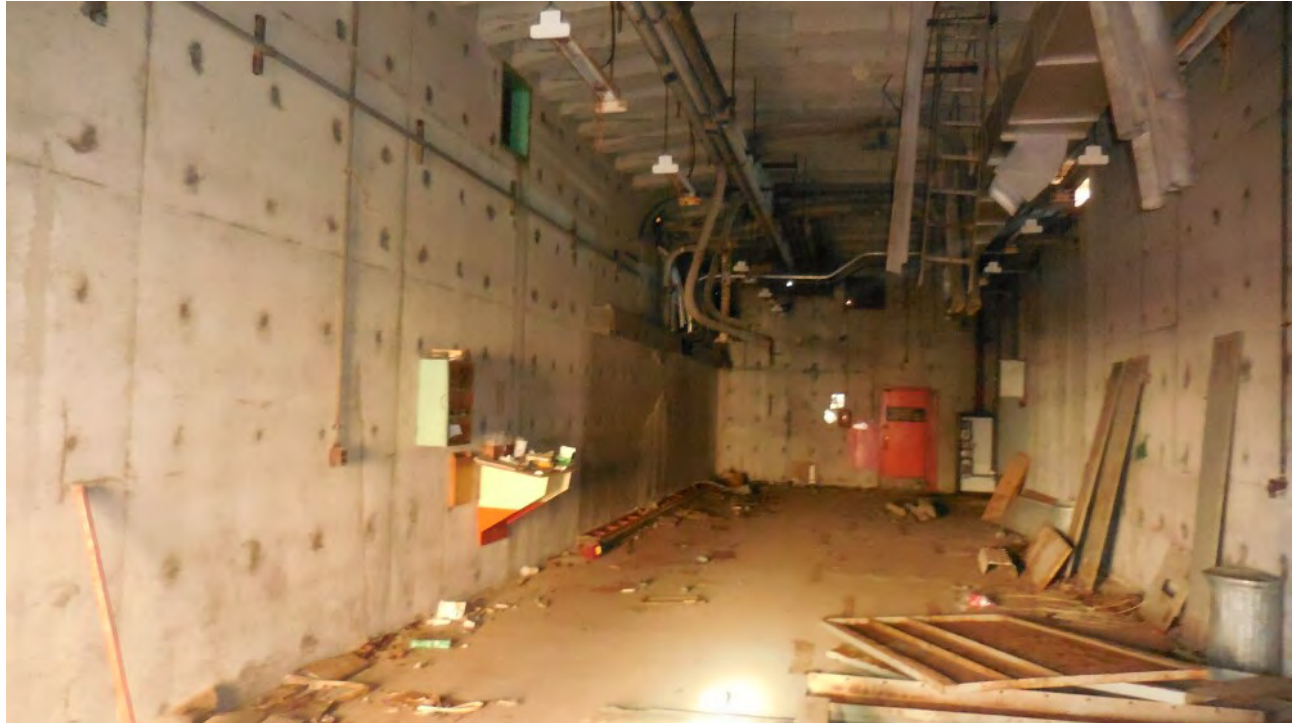
Figure 36. Interior – Structure 2. No signs of bats, but suitable habitat present in upper floor.
