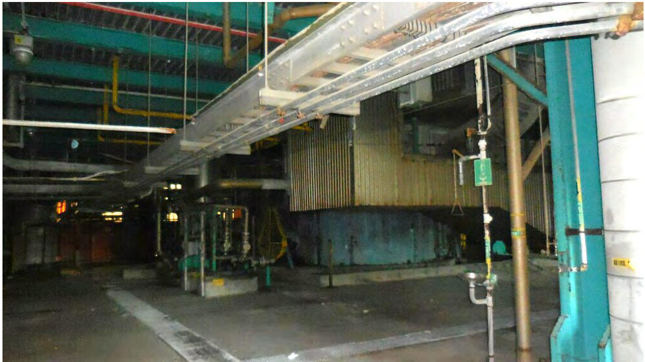
Figure 17. Interior of 12-Story Boiler Building. Large amounts of light and in some locations, airflow, not conducive to bat roosting activity. No signs of past or present use found.
