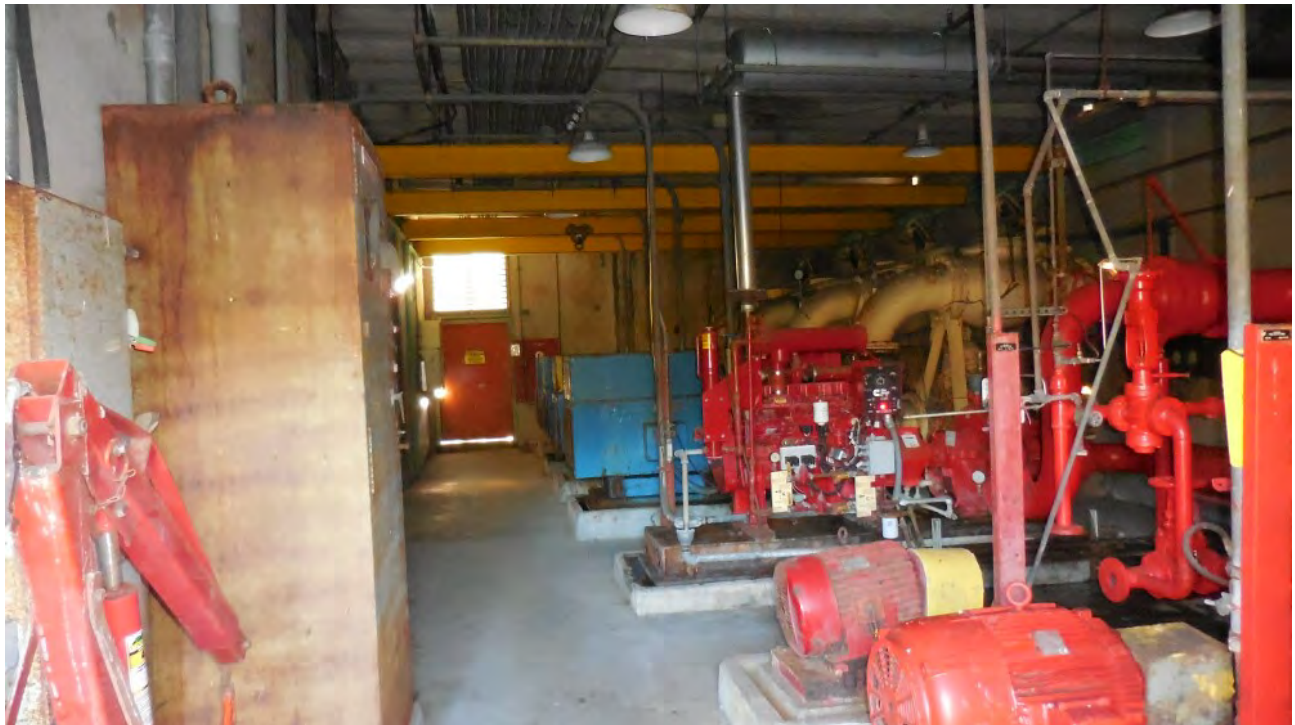
Figure 4. Interior of Pump House. Bat activity noted throughout. Remove only during seasonal periods of bat activity after conducting partial dismantling/deterrence measures as detailed in text.
