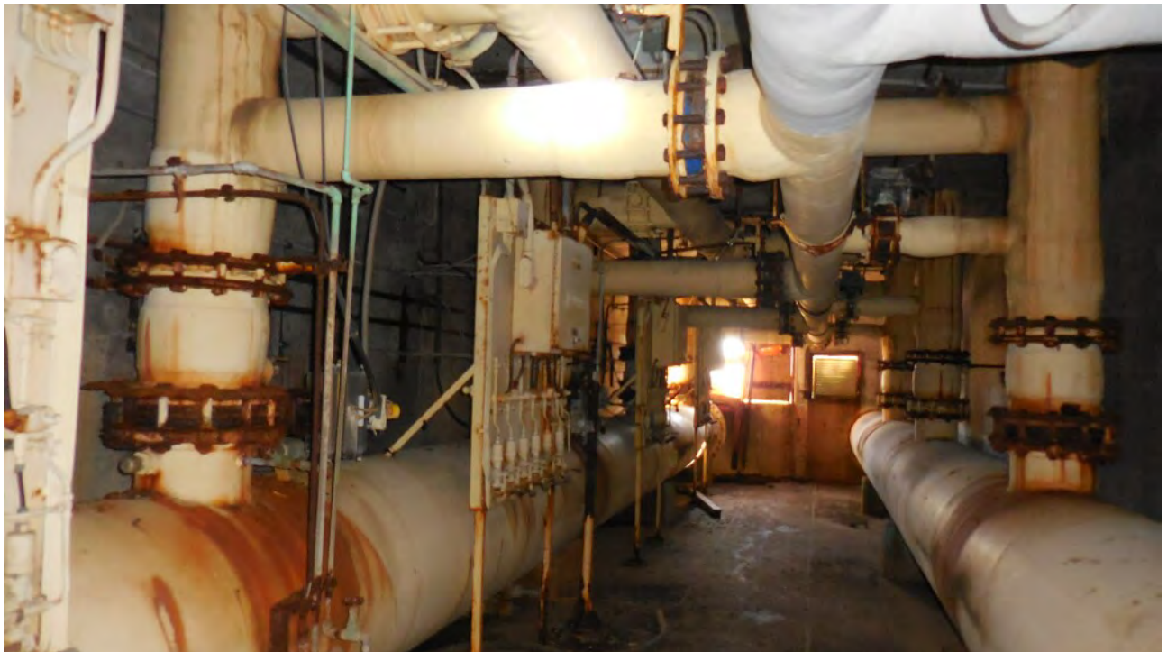
Figure 14. Interior of J-shaped Tank Support Building attached to Filter/Softener Tank Building. No signs of use by bats, but suitable potential habitat.
