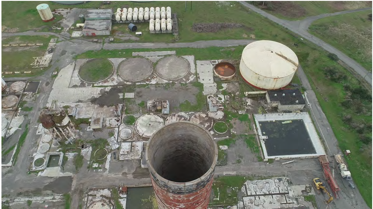
Figure 25. Open mouth of Smokestack – Unmanned Aerial Vehicle (UAV) photo by Nordic Aquafarms.
