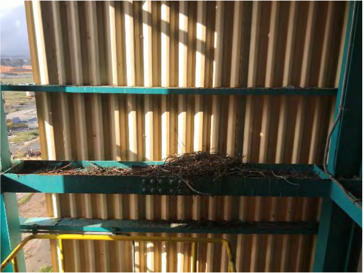
Photo 1. Inactive raptor or Common Raven ( Corvus corax ) nest in boiler building.
