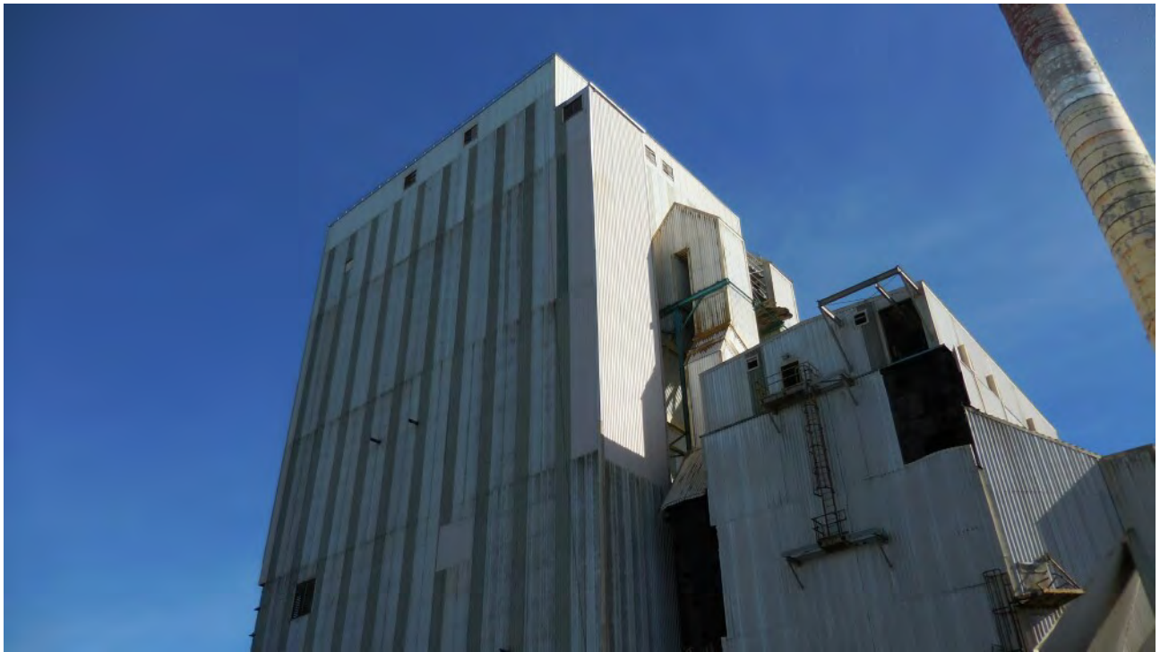
Figure 15. West-facing portion of 12-Story Boiler Building and attached structure. No signs of past or present use by bats around exterior or interior.
