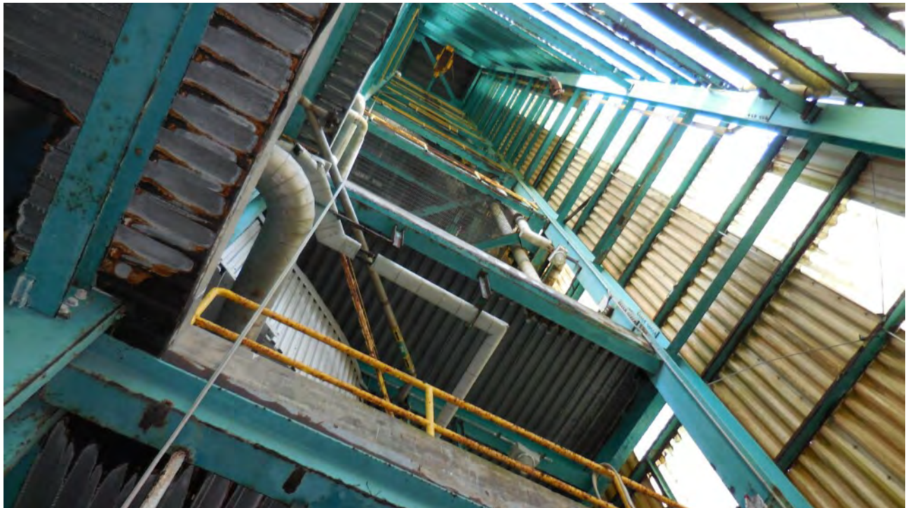
Figure 18. Interior of 12-Story Boiler Building. Large amounts of light and in some locations, airflow, not conducive to bat roosting activity. No signs of past or present use found.
