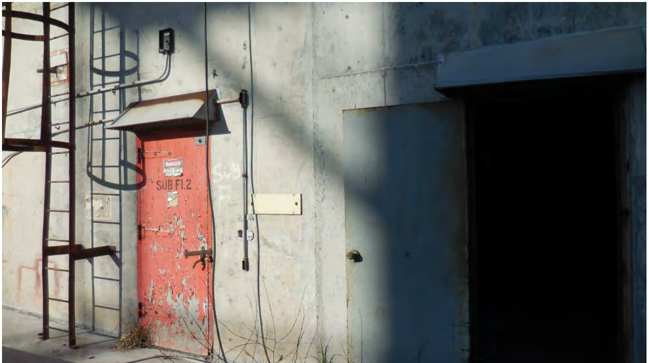
Figure 8. Building SUB FL.2. Bat activity noted in several interior locations.
