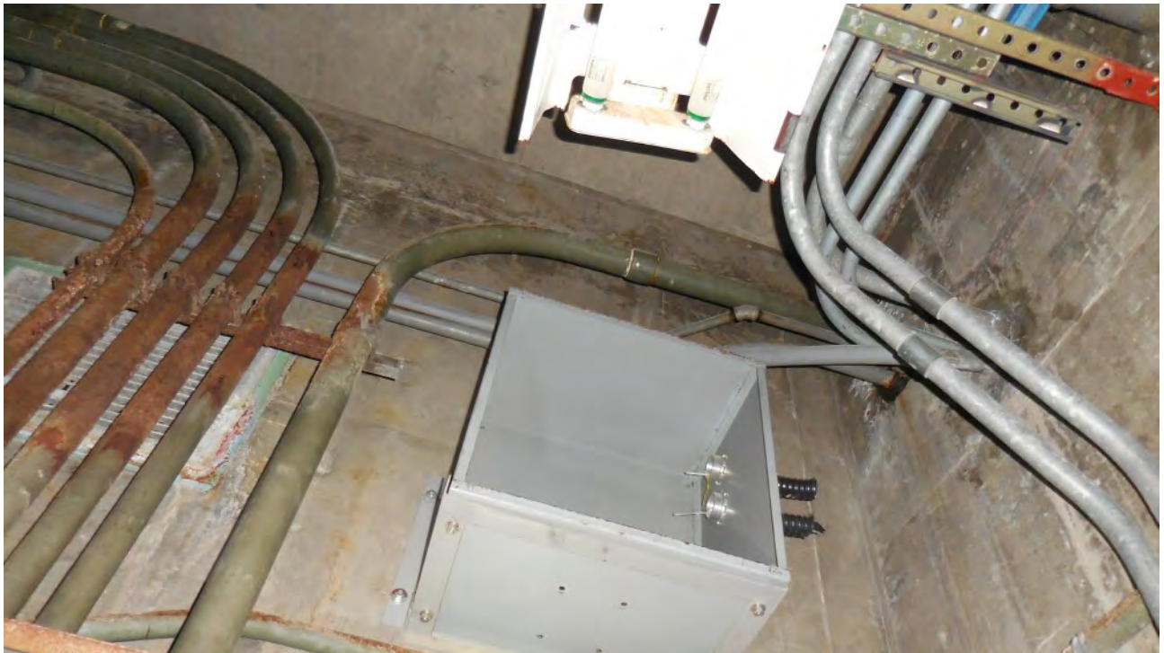
Figure 10. Building SUB FL.2. Bat activity noted in several interior locations.
