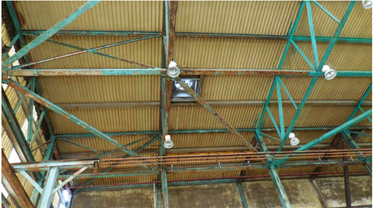
Figure 53. Interior of Machine Building – large amounts of light and airflow, not conducive to bat roosting activity.
