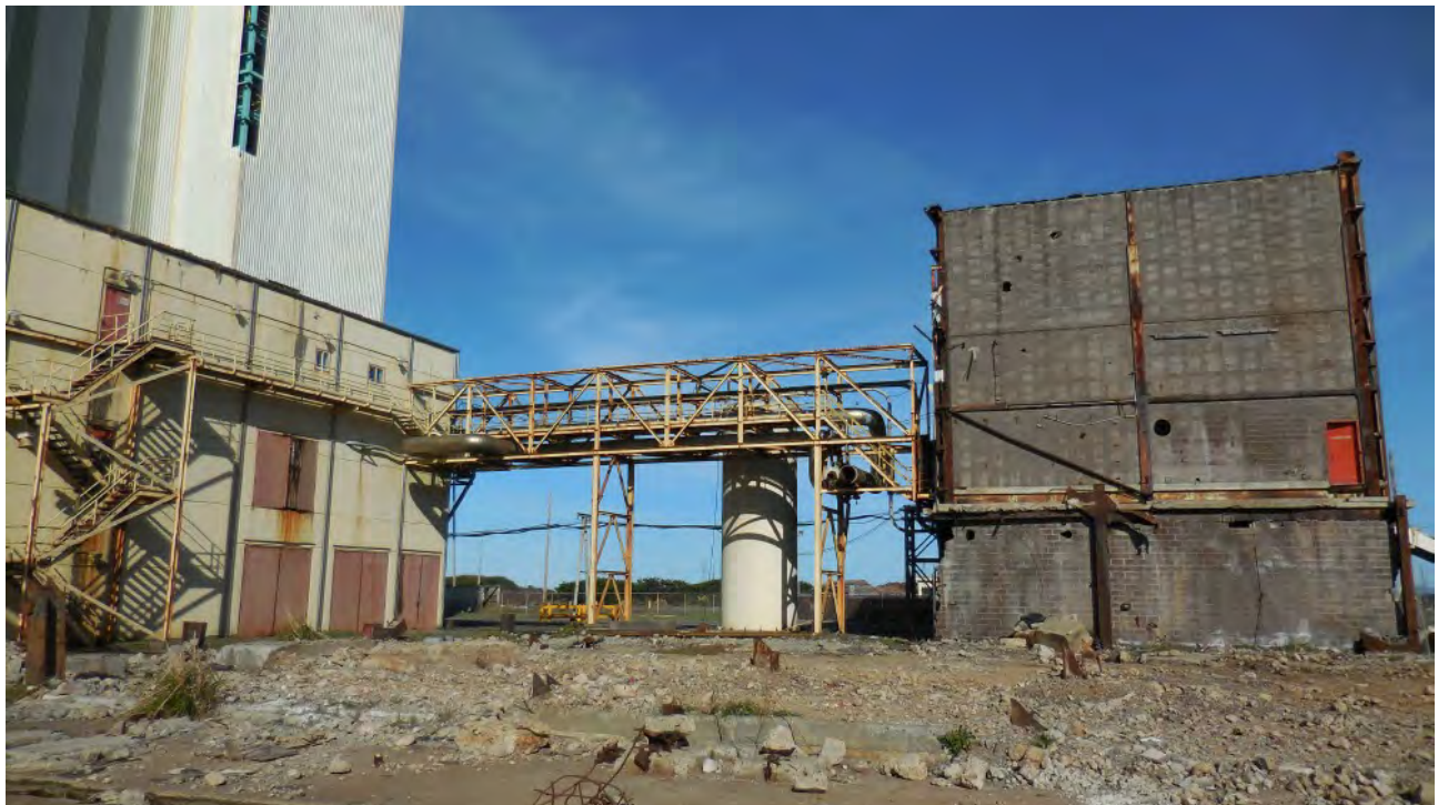
Figure 30. South-facing portion of 3-Story Boiler Building just east of 12-Story Boiler Building. No signs of bat activity, exterior or interior.
