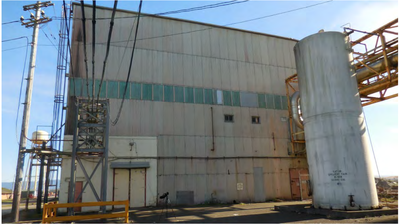
Figure 31. West-facing portion of 3-Story Boiler Building just east of 12-Story Boiler Building. No signs of bat activity, exterior or interior.
