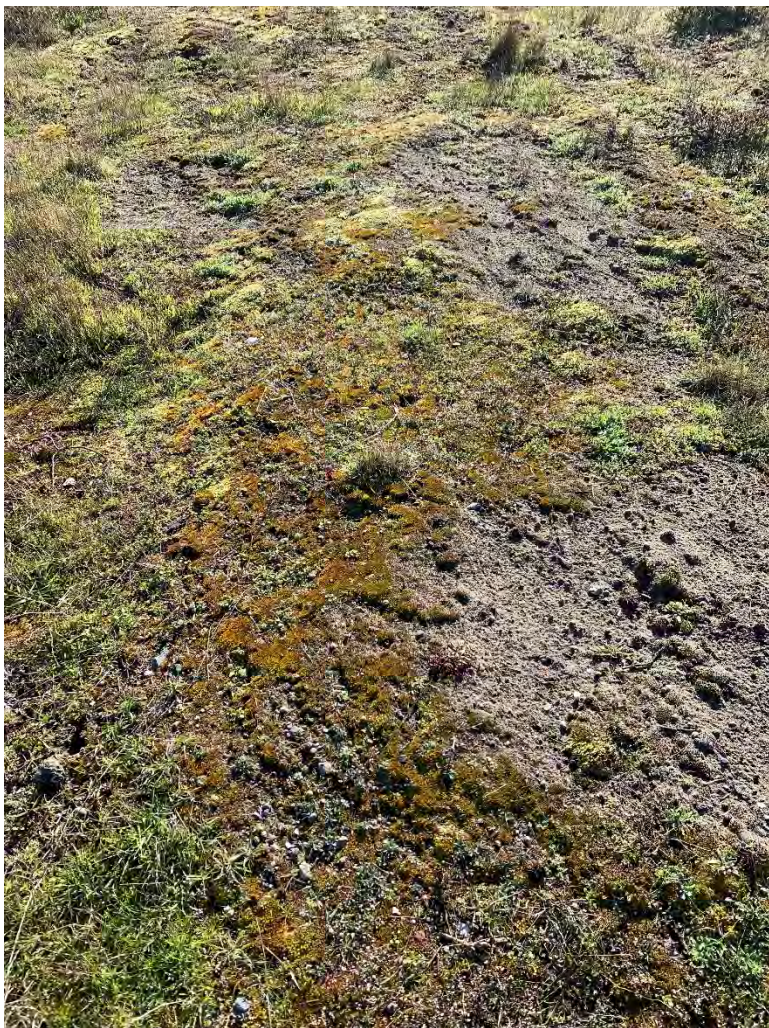
Photo 5. Scattered gravel in the access road along the fence line.
