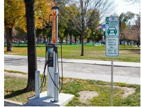
Illustrative of Electric Vehicle Charging Station
