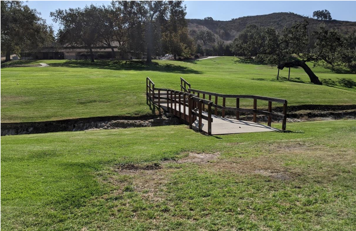
Photograph 5b. Existing bridge over creek, looking south with community center in the background
