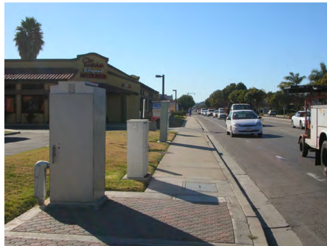
Unlike current development practices (left), utility boxes and other structures should be buried or screened to prevent impacts to the public realm.
