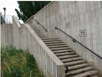
Structural flood control improvements such as stoplog structures and flood walls should be designed to be attractive as well as functional.
