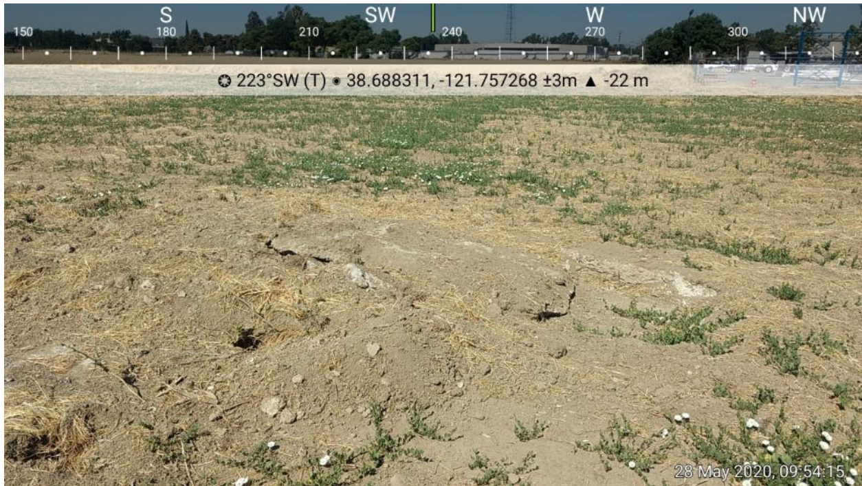
Photo 9: An example of concrete debris from former storm drain infrastructure present within the western side of the Project site, looking southwest.
