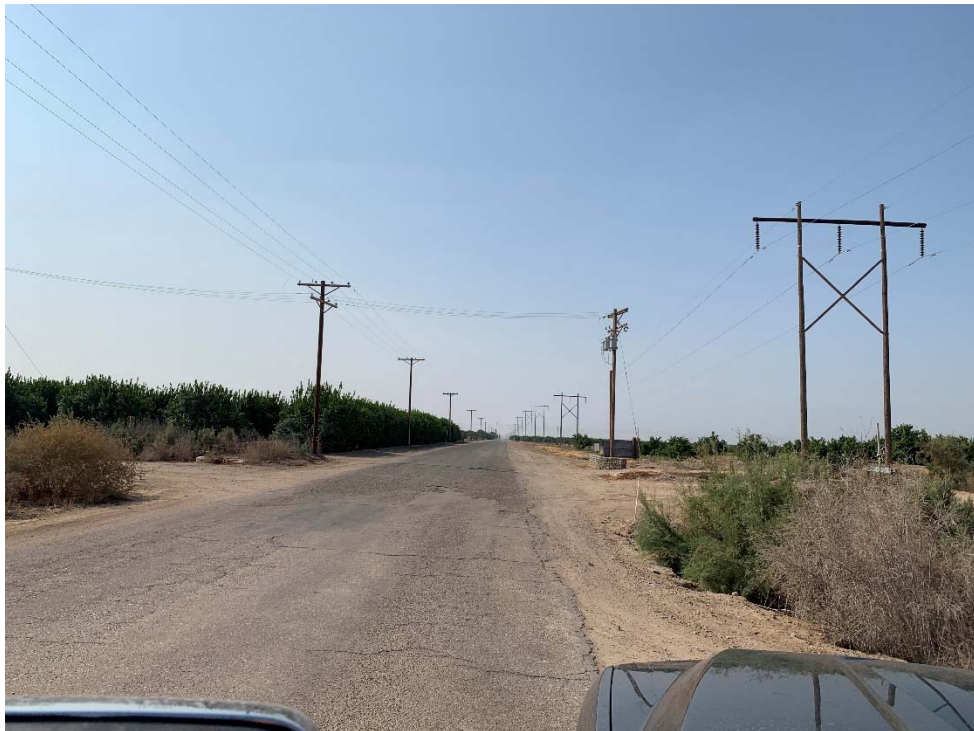
Photo 8: Looking at the IID pole mounted transformers located across Weist Road west of the southwest corner of the subject site.
