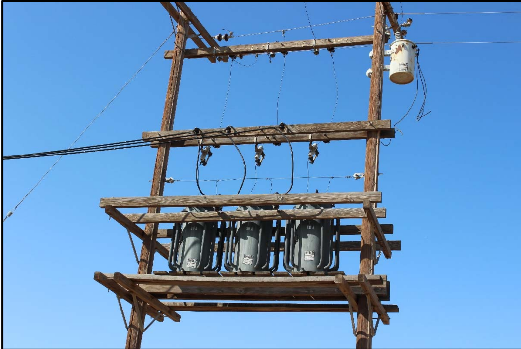
Photo 9: Close-up view of transformer bank. IID stickers show the transformers have been tested for PCBs.
