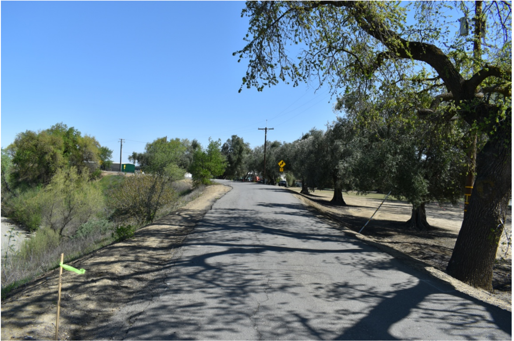
View of levee restoration project area on top of County Road 18, facing east (March 2021)
