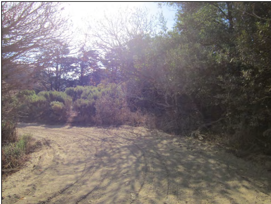
Photo 2. Location where drainage feature crosses existing dirt driveway (via culvert), approximately 370 feet west of driveway entrance, view east. September 27, 2018.
