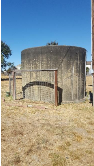
Subject Property - cement water tank
