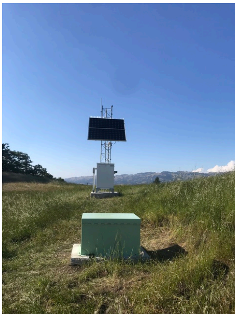
Photo of typical EEW installation.
