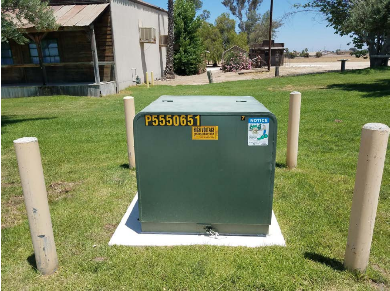
Pad mounted transformer, owned by Edison.
