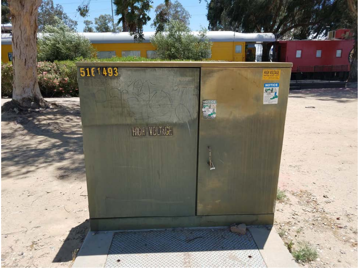
Another pad mounted transformer.
