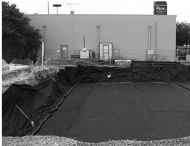
Place non-woven geotextile over prepared soils and up excavation walls. Install underdrains if required.
