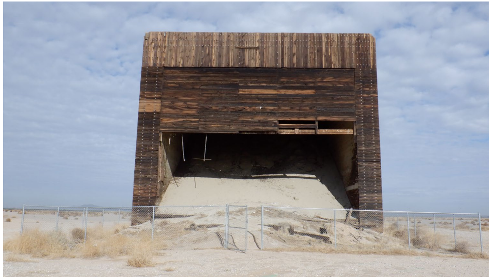
Photograph 13. View northwest of southeast facade of Facility 811. Note the interior earthen mound intended for live munitions fire from military aircraft.
