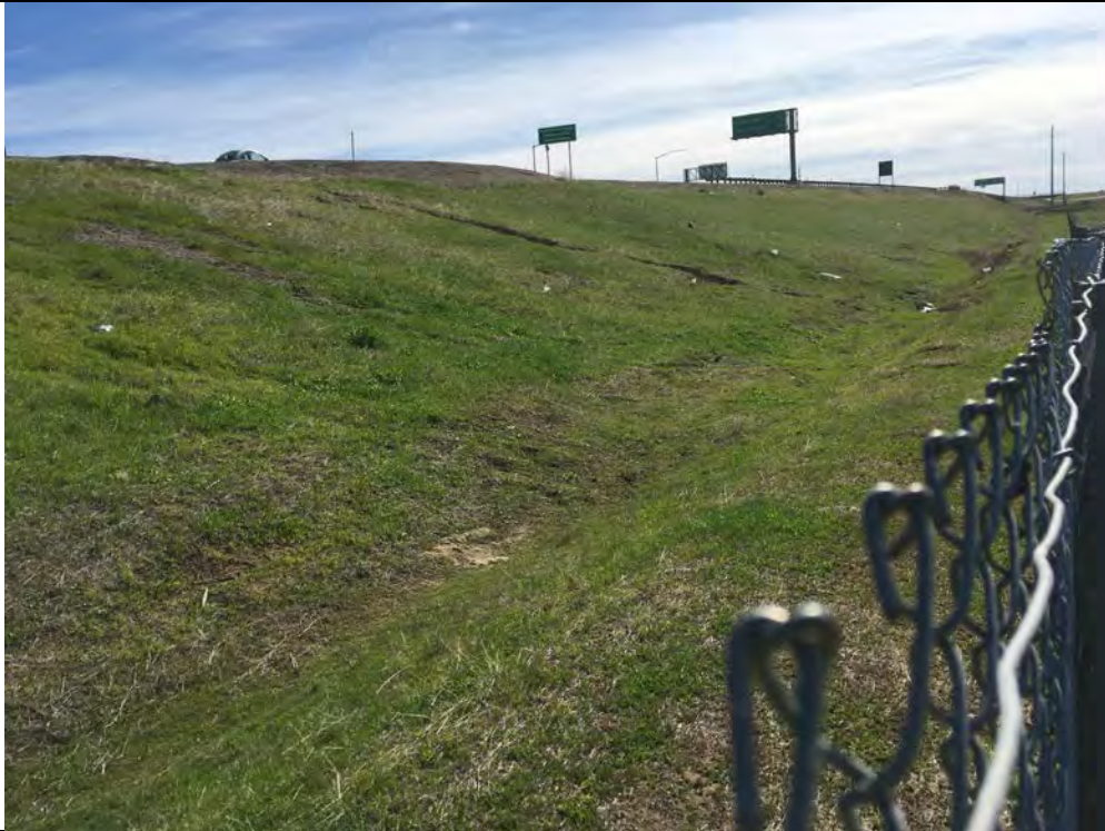
13. Facing southeast, the photo depicts the offsite roadside ditch just east of the Property, which flows parallel to Highway 4. This feature did not contain water during the time of the survey.
