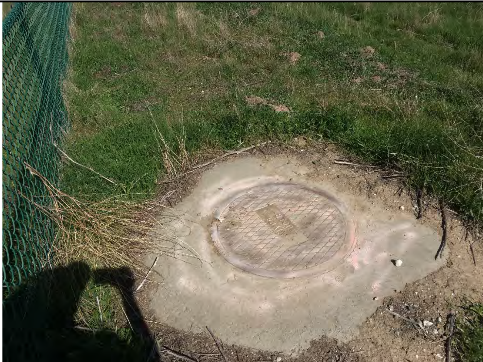
10. The photo shows one of the stormwater manhole covers present along the western boundary of the Property.
