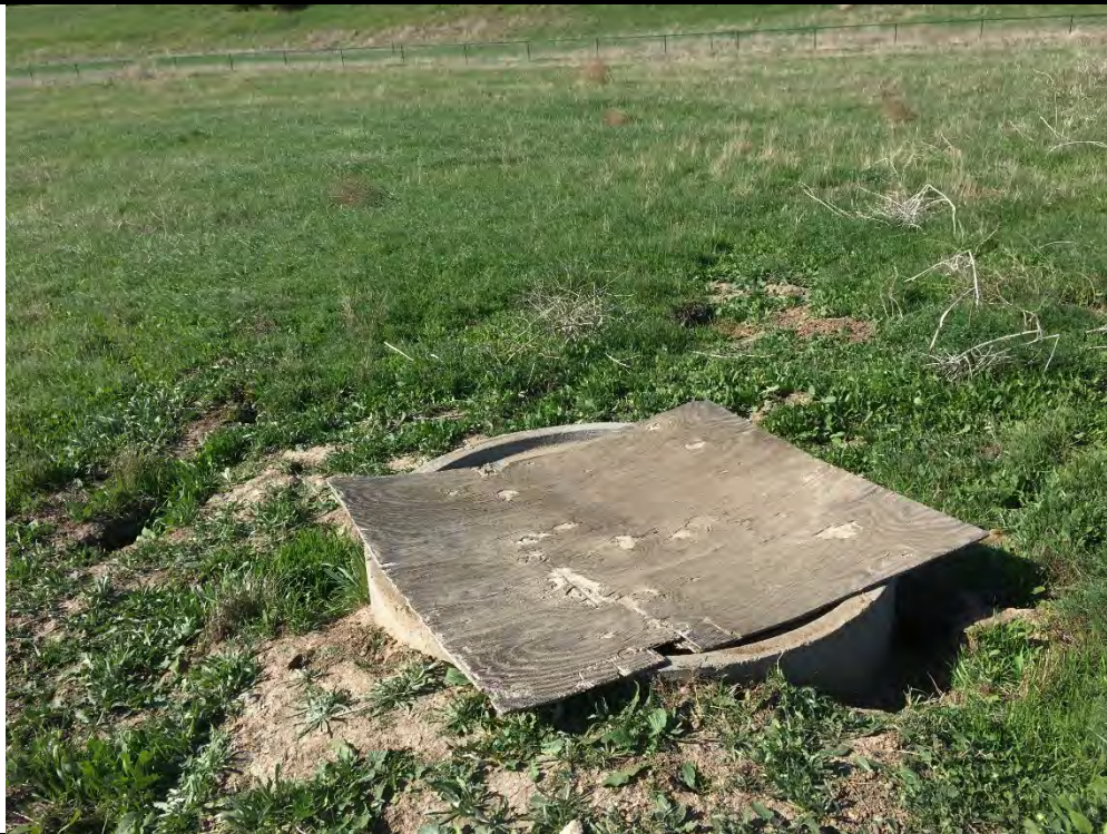
11. Facing west, the photo depicts a concrete storm drain base located in the center of the Property.
