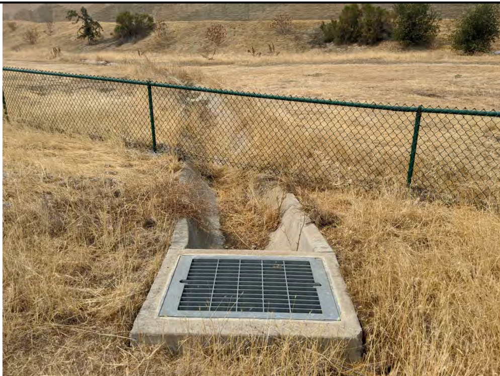
4. Concrete v-ditch enters the northern end of the Property and flows to this stormdrain. Taken August 2020.
