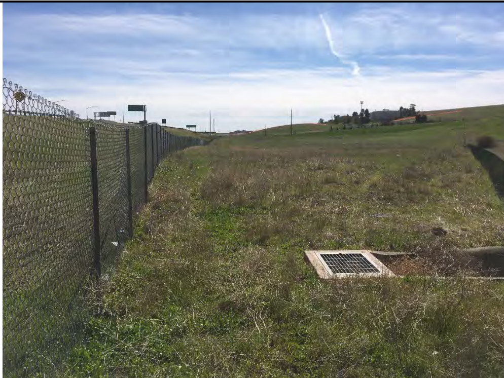
12. Facing south from the northernmost tip of the Property, the photo shows the concrete v-ditch and storm drain present at the northern end of the Property.
