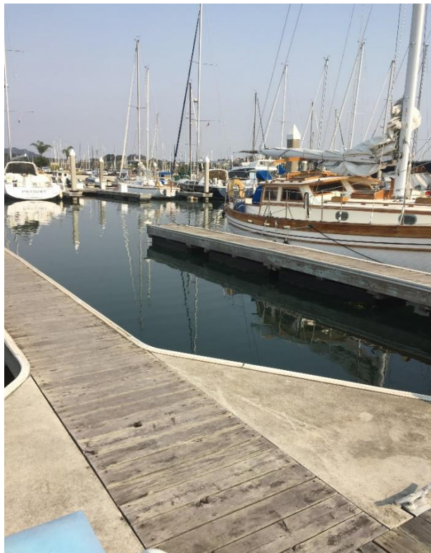
Photo 6. View of Basin 3 dock slip, with dock freeboard, looking north. (MIG site visit, 9/29/2020)
