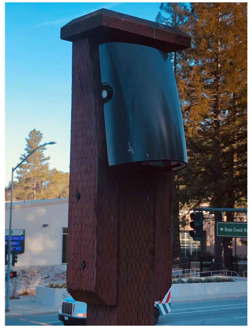
NOTE: LIGHT FIXTURE INTEGRATED IN 8' TALL FENCE POSTS OR AFFIXED TO BUILDING.
