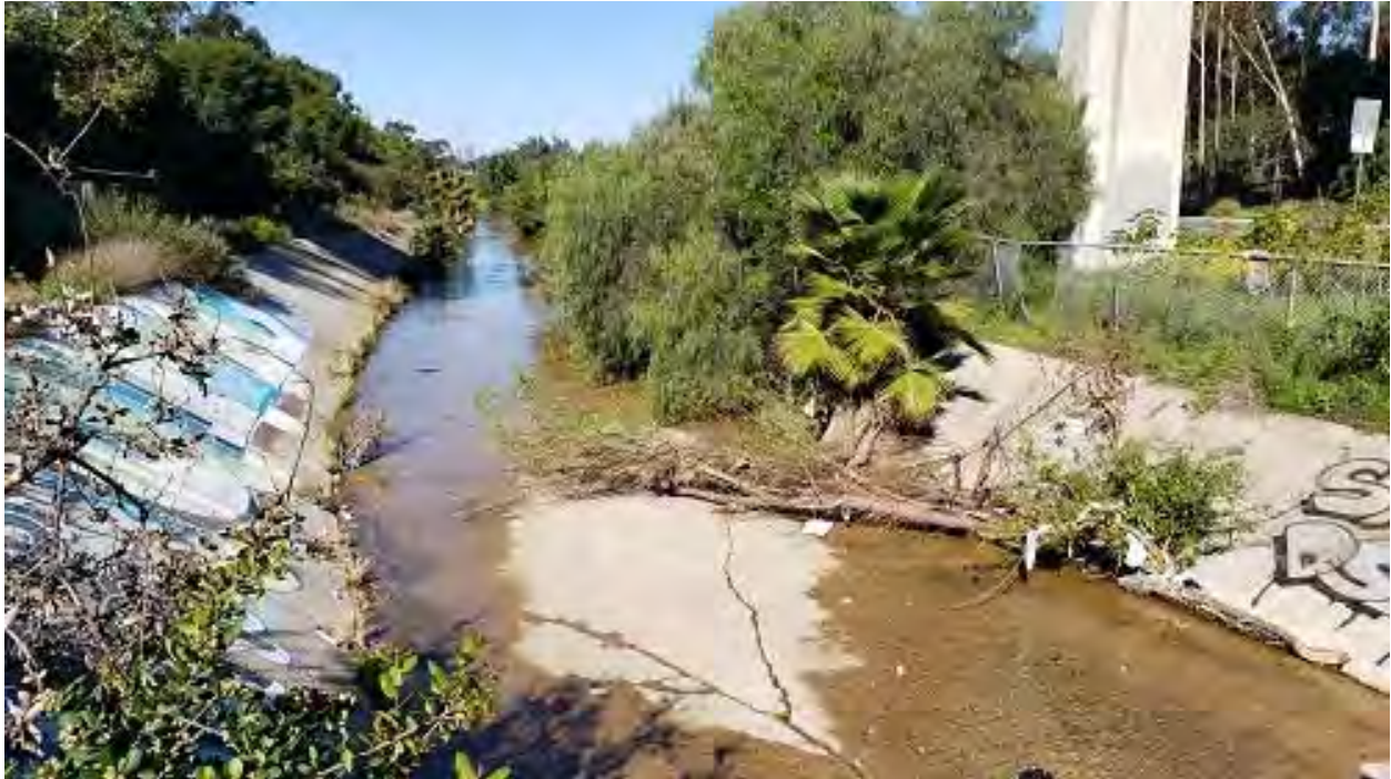
Photo 1: View of Chollas Creek from upper end of Project. Concrete removal will begin downstream of the I-805 Bridge piling, as seen on the right of the photo.
