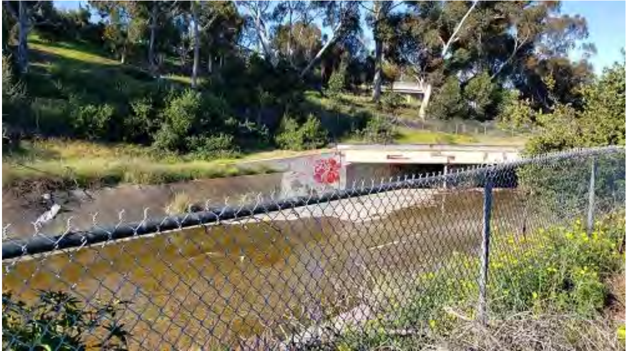
Photo 5. View of bridge structure that will be removed as part of the Project, looking downstream.
