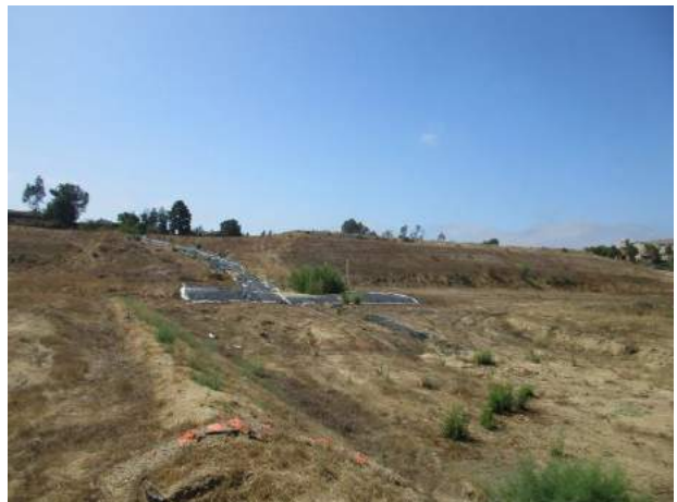
12. Additional view of the stormwater management installment on the central portion of the property.
