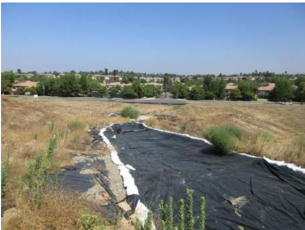
11. View of an engineered erosion prevention best management practice installment on the northern-central portion of the lots.
