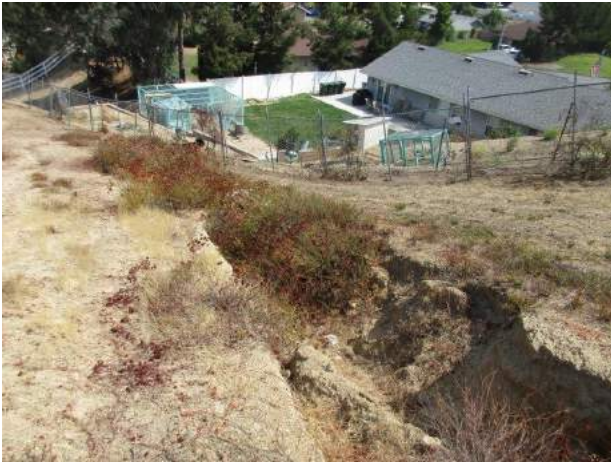
13. View of a large erosion channel on the south-eastern side of the subject property.
