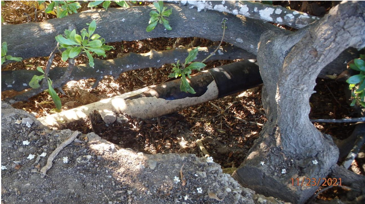
Asbestos Survey Partially Exposed 6-Inch Diameter Steel Pipeline along Pier Access Road PRC 421 Decommissioning Project, Goleta, Santa Barbara County, California
