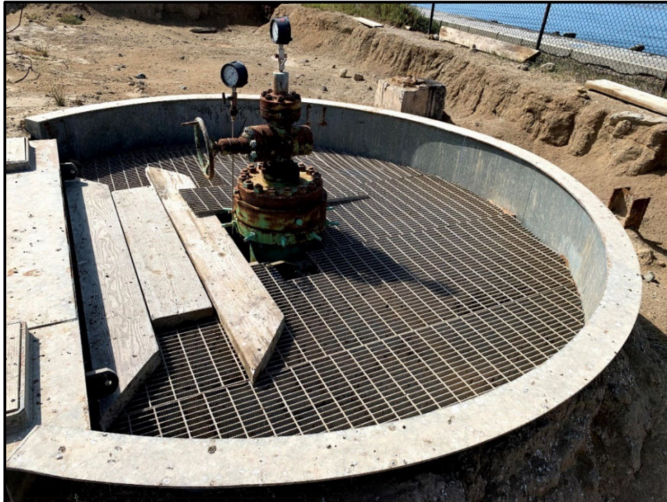
Figure 2-8. 421-2 Well Riser (Within Concrete Cellar Ring)
