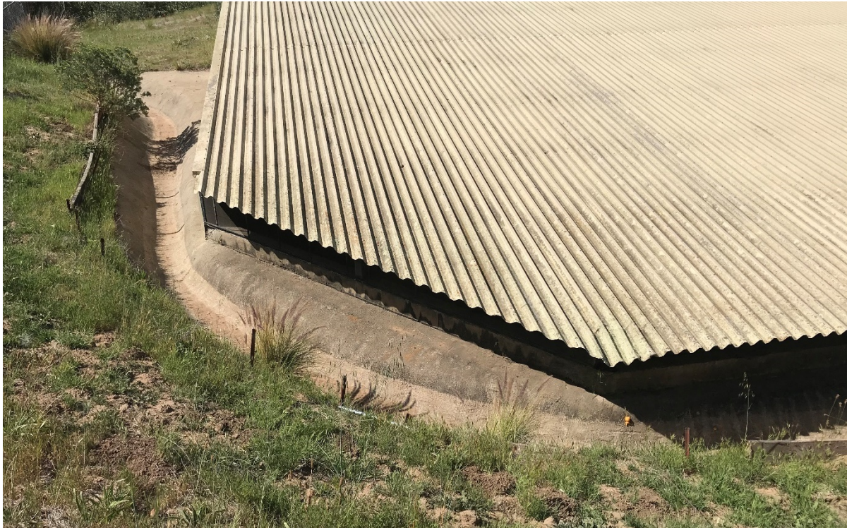
Figure 36 East End of Romero Reservoir, Including the Outlet Channel, View to the South
