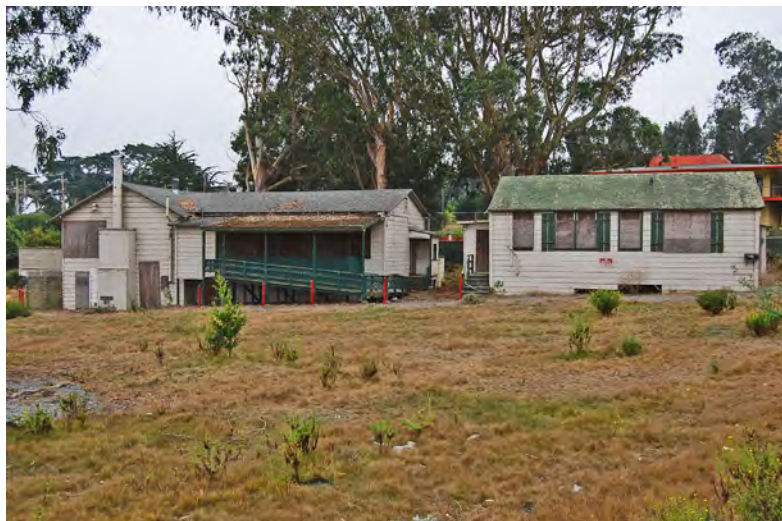
Photo 1. Clubhouse on left and Caretaker's House on right; facing south; (contributing features)
