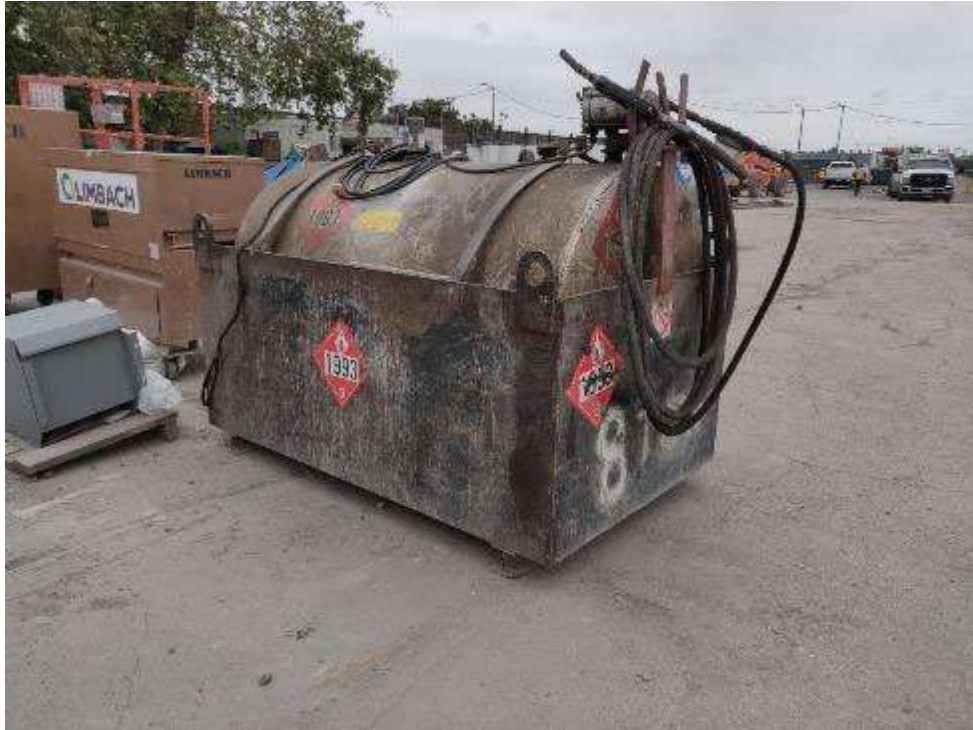
Photo 7: Diesel fuel AST on the East Block used for vehicle fueling
