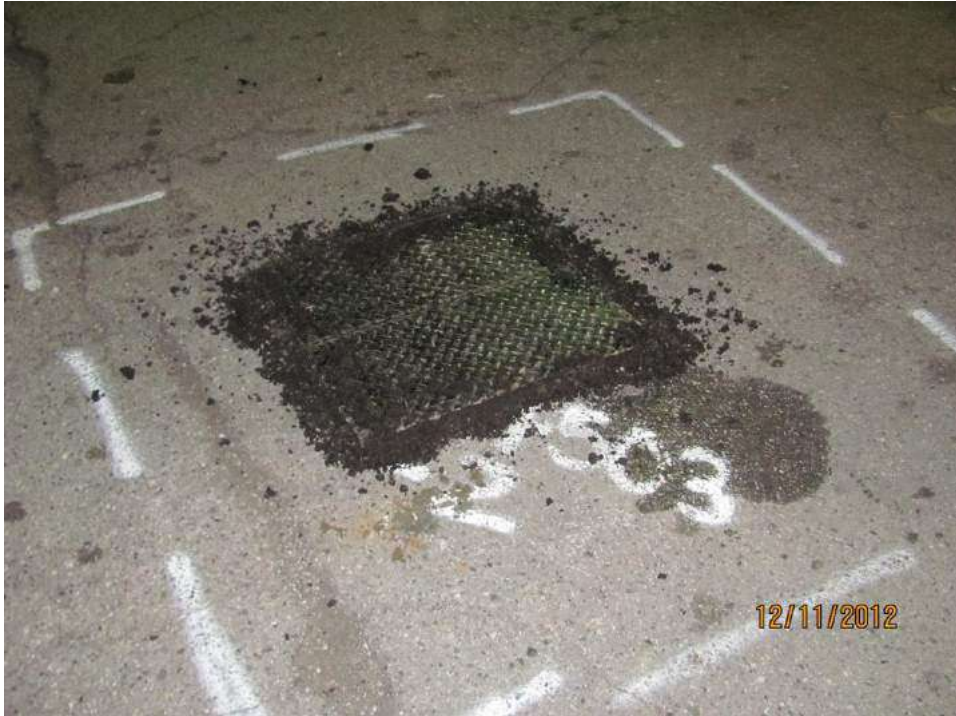
Temporary metal cover on nested soil gas probe location
