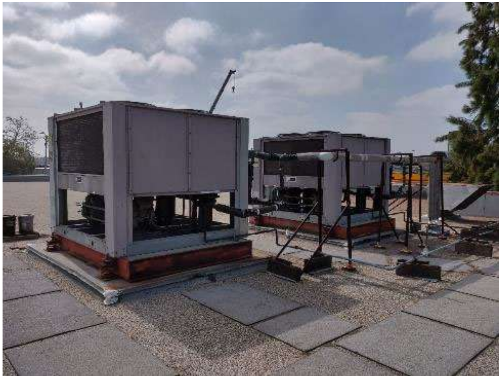
Photo 16: Two rooftop cooling towers at the LA Probation Building (West Block)
