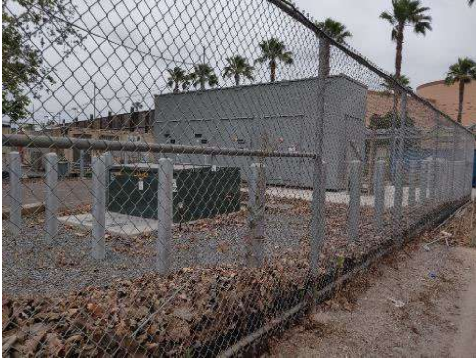
Photo 11: One of two pad-mounted transformers on the East Block
