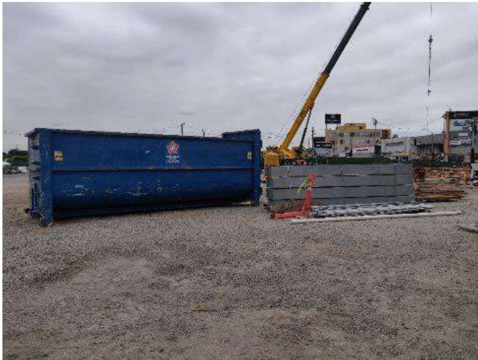
Photo 10: Industrial-sized roll off waste bin on the East Block for disposal of construction-related wastes
