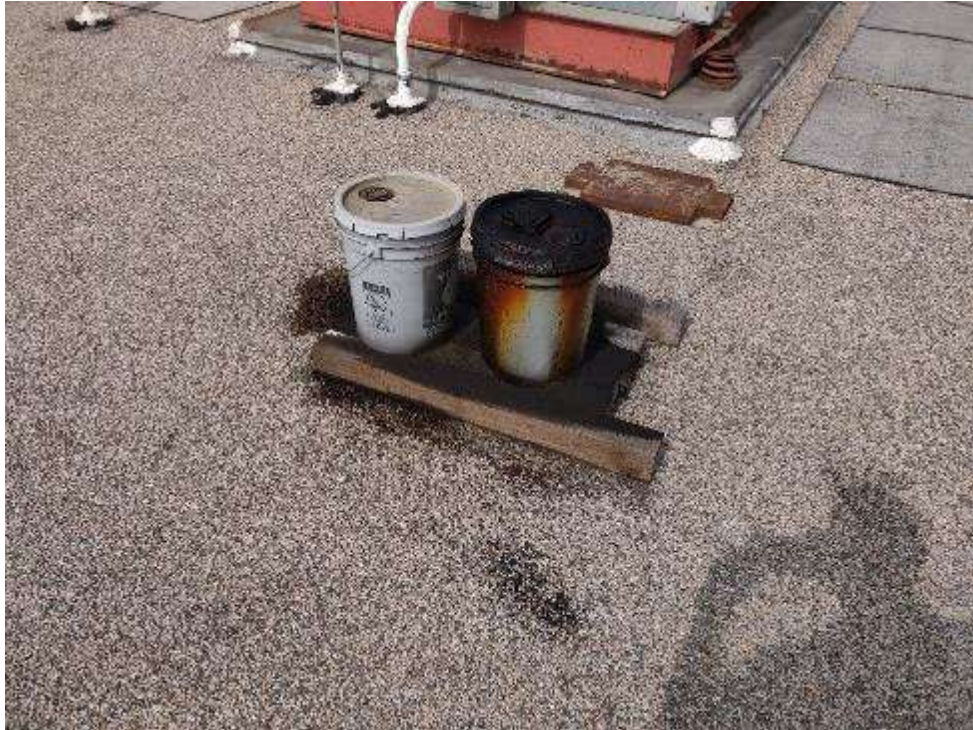
Photo 17: Oil containers with associated de minimis visible staining on the roof of the LA Probation Building (West Block)
