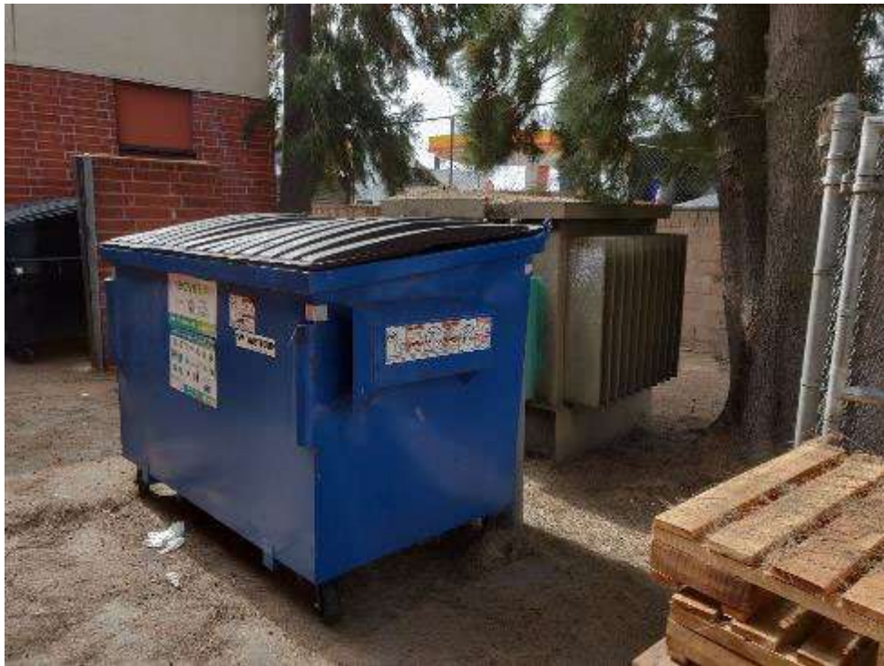
Photo 20: Open-top dumpsters and a pad-mounted transformer near the southwestern corner of the LA Probation Building (West Block)
