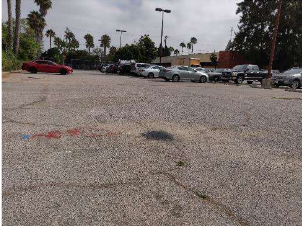
Photo 13: View of the West Block's parking area with an abandoned soil boring in foreground
