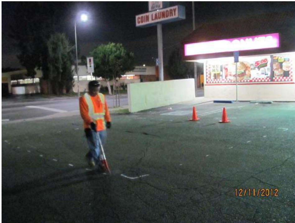
Area of disturbed subgrade soil that is suspected to be a former UST location
