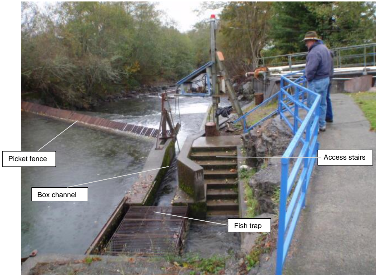
Image 1-2. Fish Trap (looking downstream from river right) and picket fence in upright position
