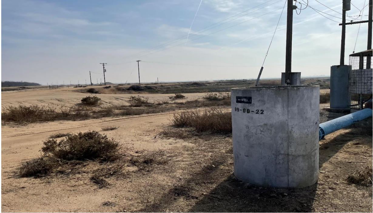
Photo 7. Well 99-00-022 adjacent to Rosedale spreading area (facing southwest).
