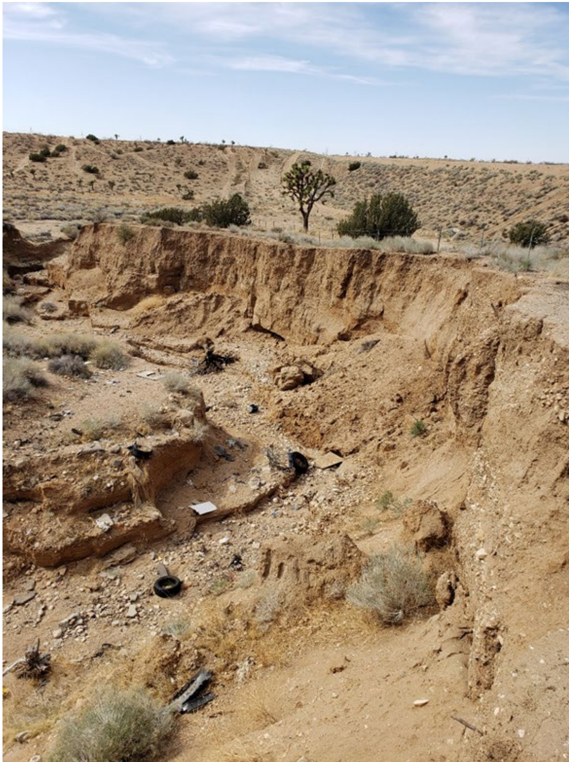
Attachment 2. Erosion channel scoured downslope of Cataba Road storm drain with the Aqueduct embankment in the background.
