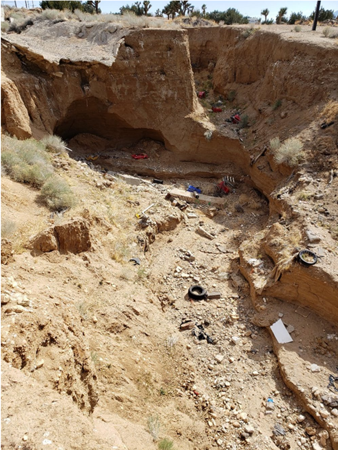
Attachment 1. Erosion immediately downslope of Cataba Road storm drain concrete discharge apron.
