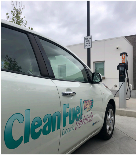
Electric Vehicle Charging Station
