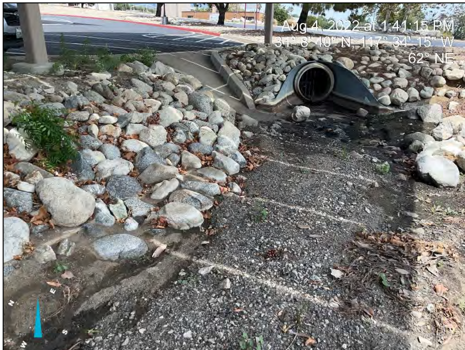
Looking east at Drainage B at the storm drain inlet and curb cut.
