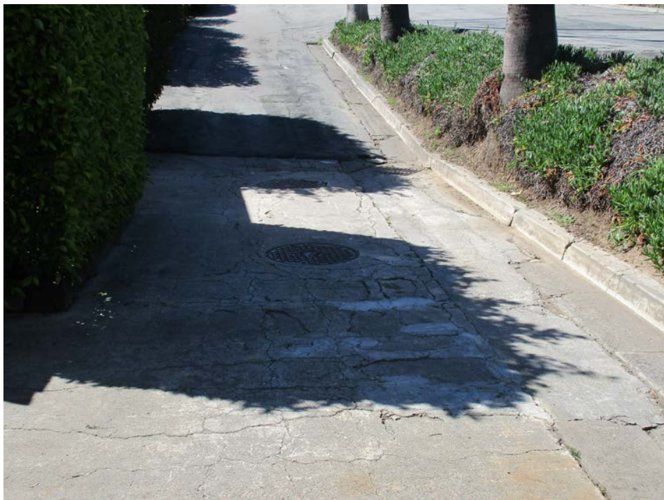
Photo 12 – Sewer manhole covers southwest of the clubhouse.
