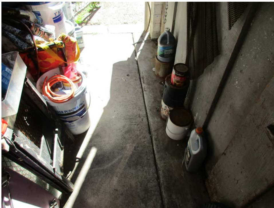
Photo 10 – Paints and lubricants adjacent to transformer cage.
