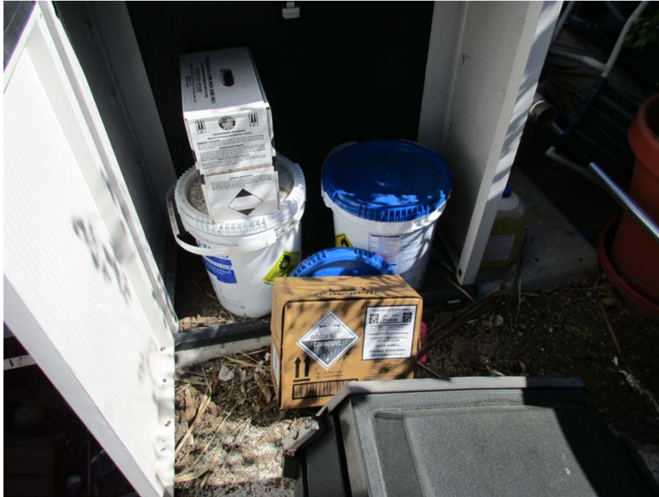
Photo 9 – Chlorine and muriatic acid storage at pool pump area.
