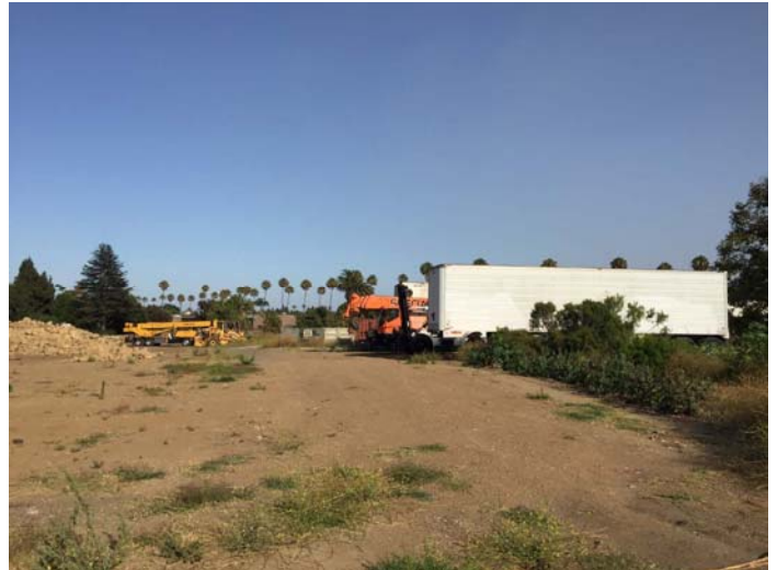
Photograph 4. Project site, looking east at location of approved apartment building (currently under construction).
