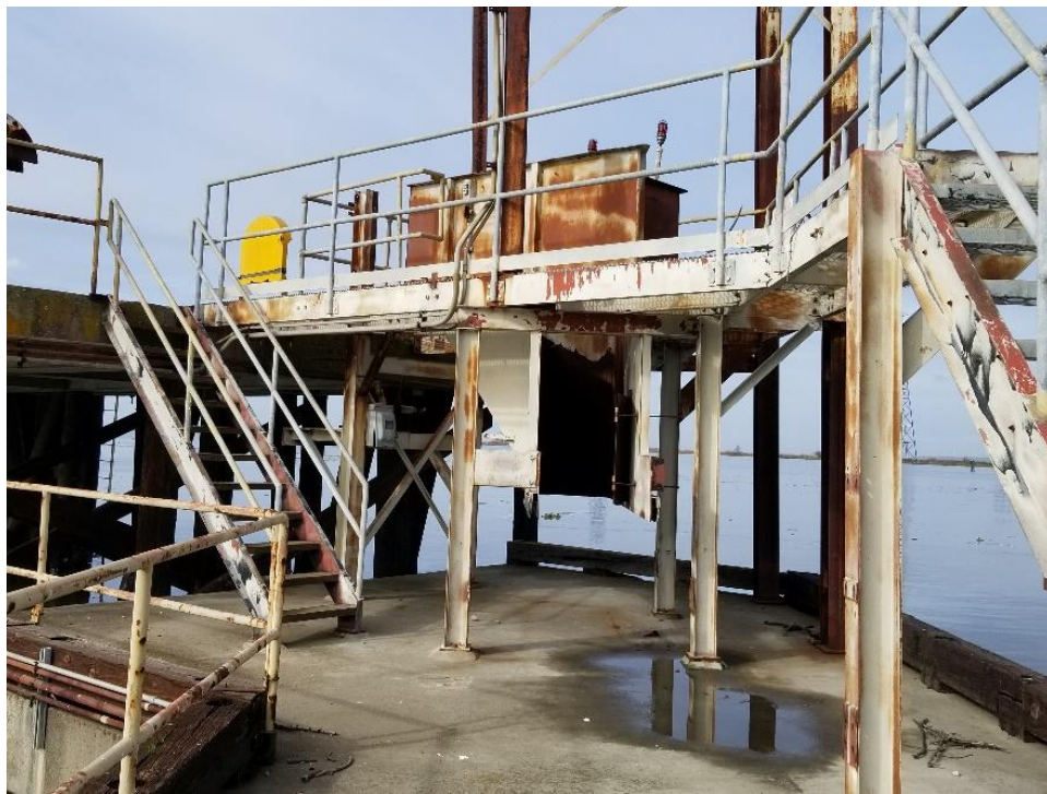
Figure 8. Hopper from upper to lower deck. Conveyor ran directly toward the camera on its way to shore.
