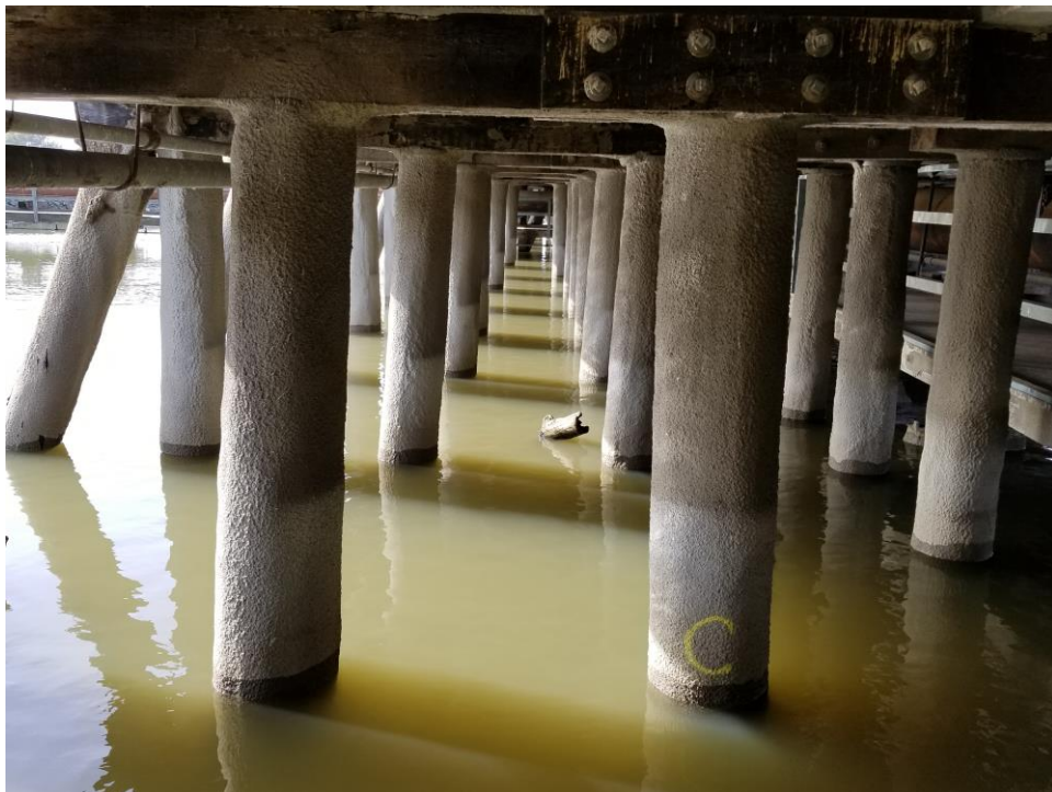
Figure 4. Piling system beneath main deck. Timber piles are covered with shotcrete for fire resistance.
