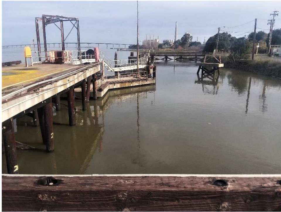
Figure 7. View from trestle toward addition at the east end of the dock and reconfigured walkway to mooring docks.
