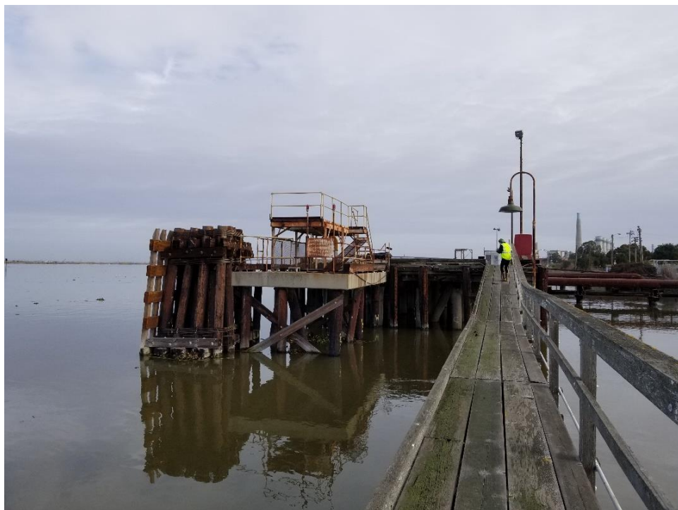
Figure 6. View toward main wharf area with Breasting dolphin at left and adjacent 1968 addition.
