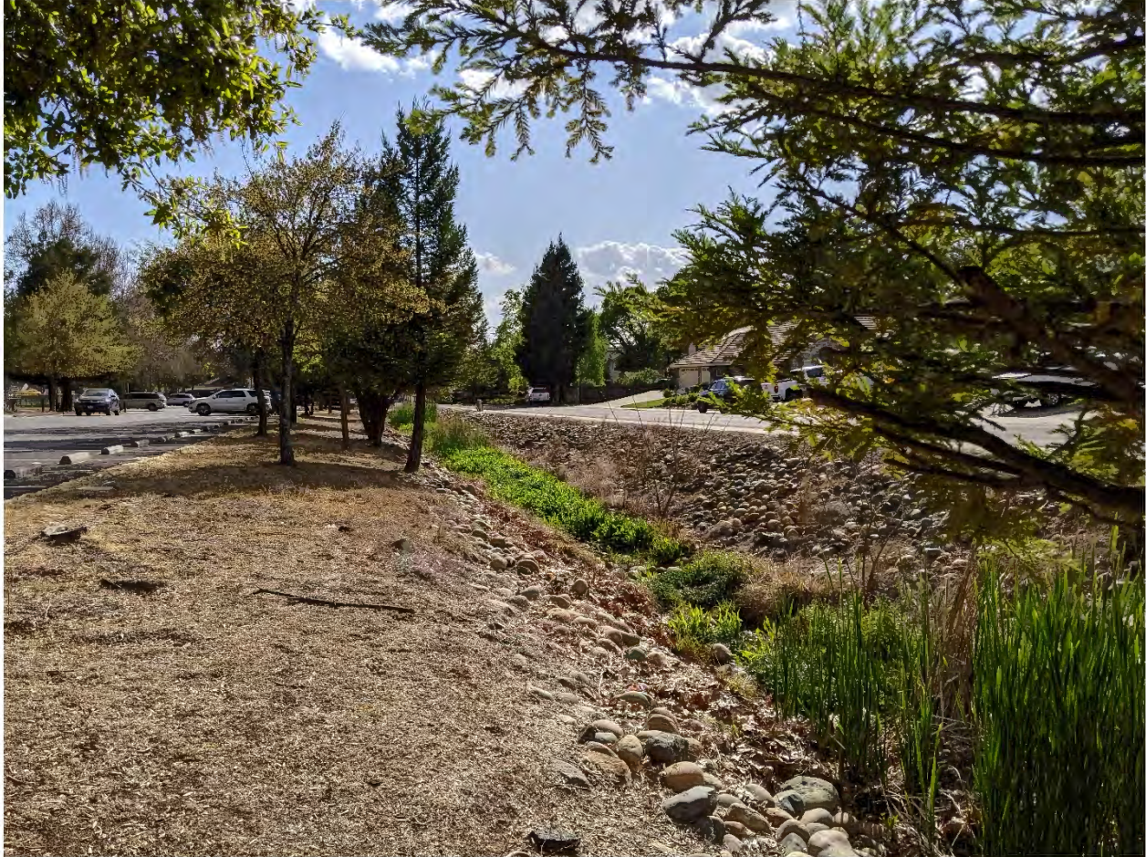
Photograph 4. Drainage on the northwestern side of the park between the parking area and Mira Loma Drive
