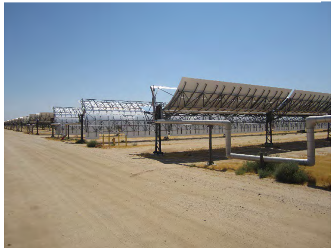
View of the SEGS IX solar fields adjacent to the south of the Project Site.
