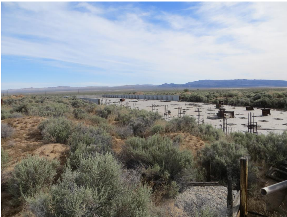
Photograph 6 – Facing northeast at a portion of the center of the project site, where existing concrete foundations and structures are present from circa 1990-1991 when this area was originally under construction but was abandoned due to funding.
