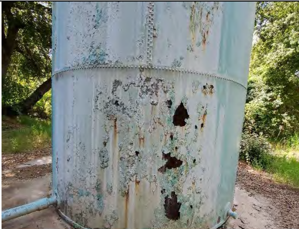
Figure 3. Rusting on exterior of tank
