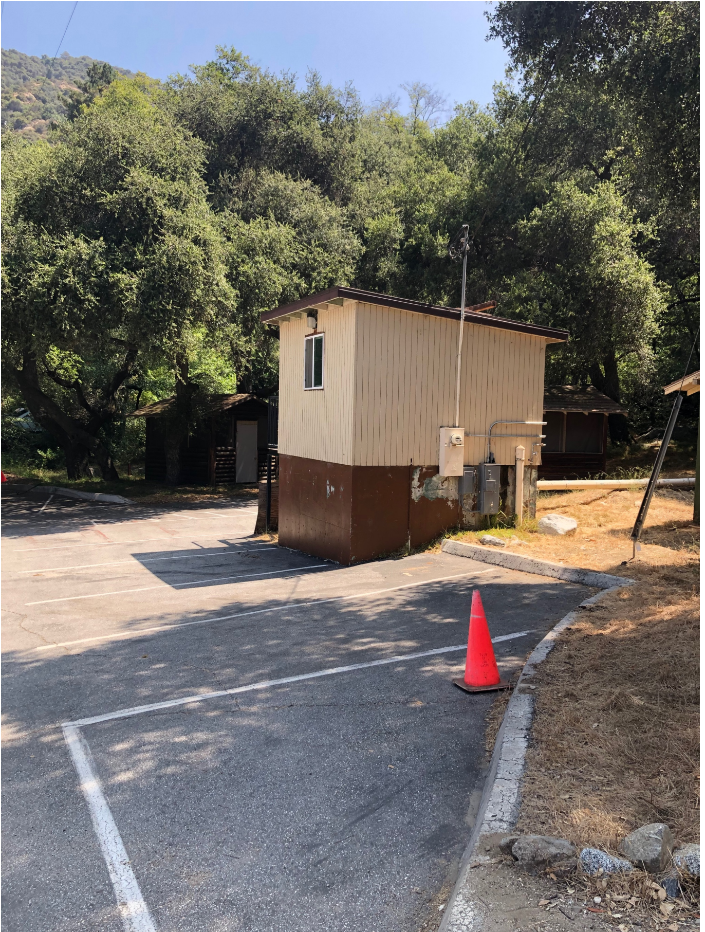
Photo 13: pump house, pump station and clearwell
