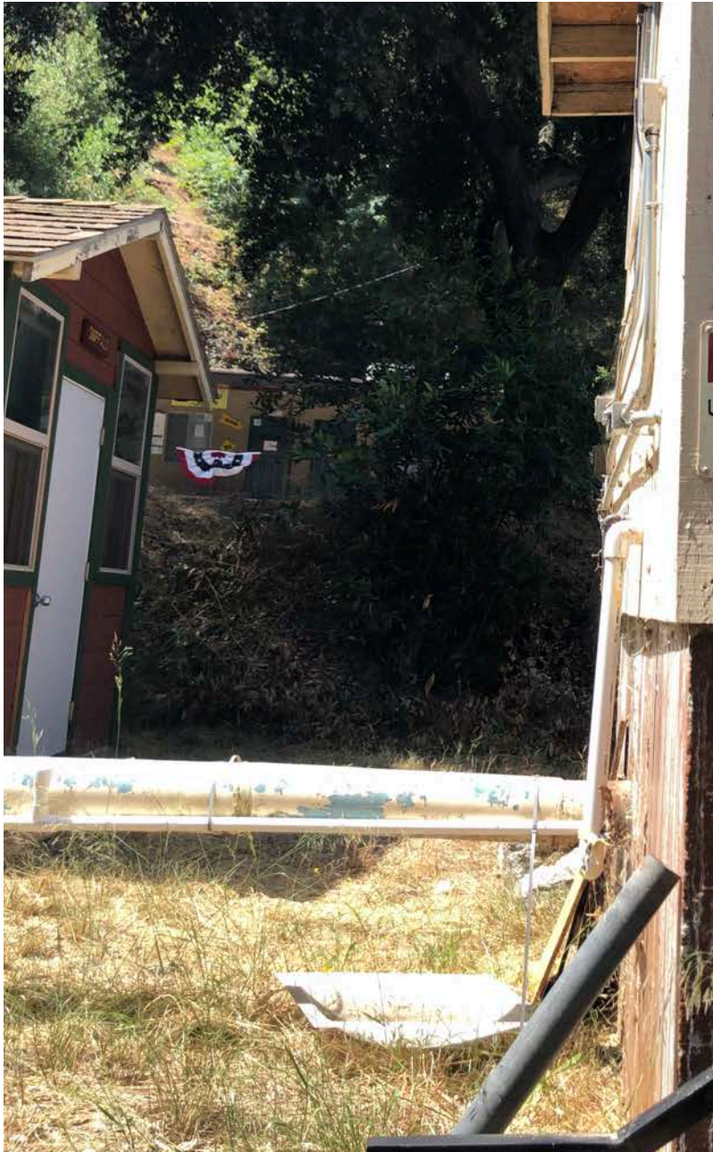
Photo 15: Pipeline connecting to pump house, pump station and clearwell
