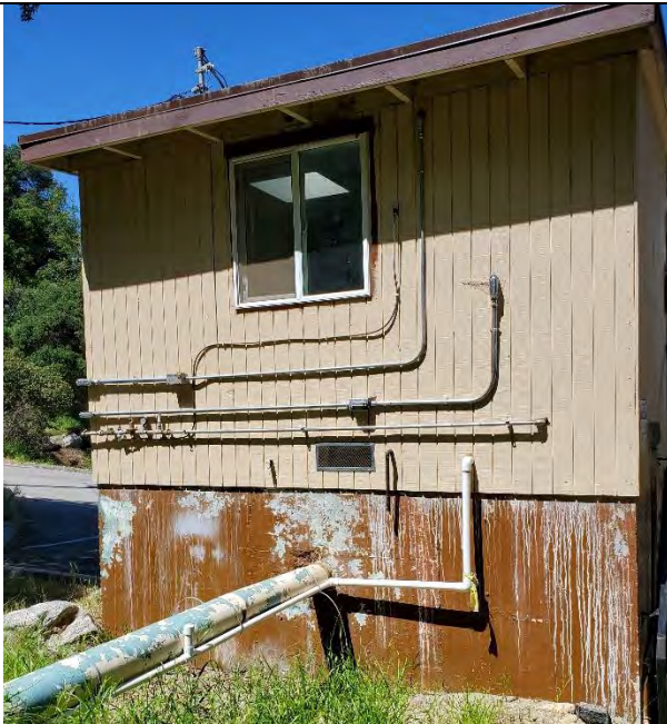
Figure 1. East side of clearwell / pump house with inlet pipe into clearwell
