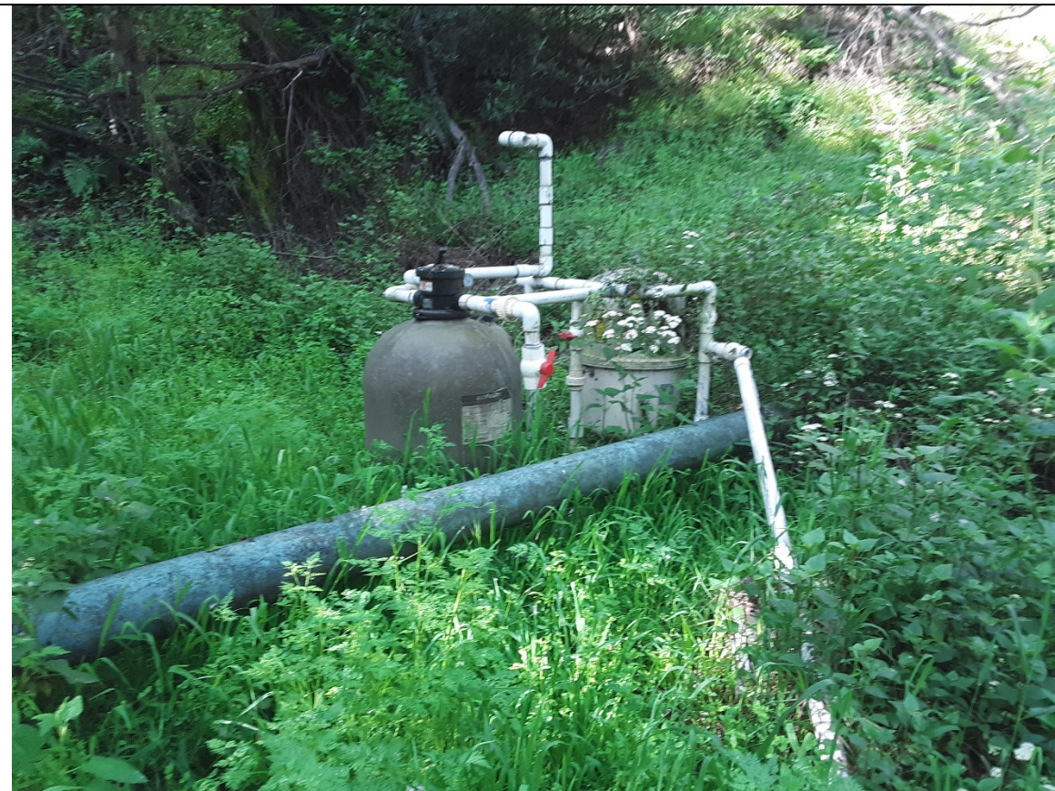
Photo 5. Pre-treatment system W (downstream) of existing intake structure.
