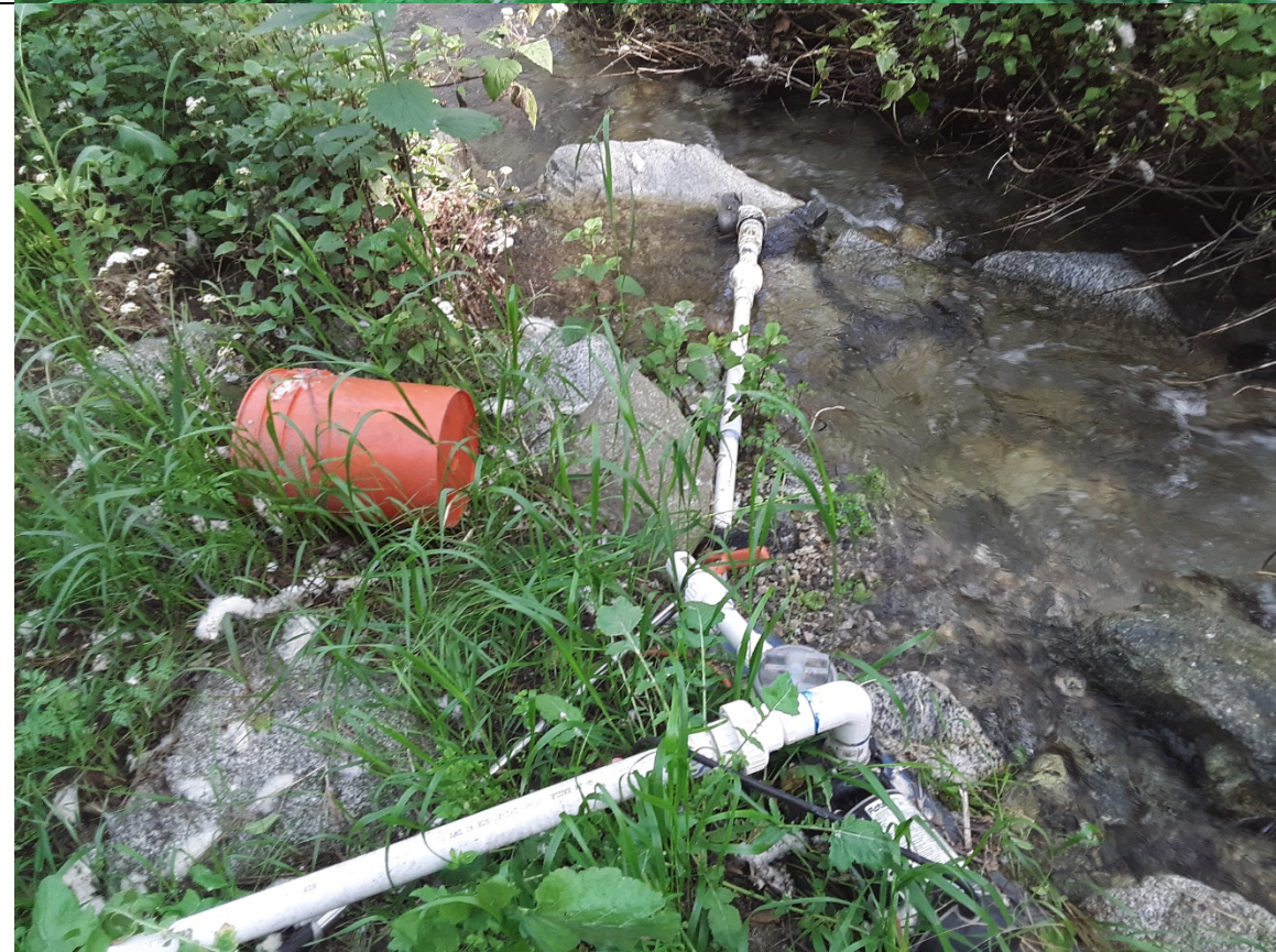
Photo 6. Temporary intake (to be removed) located W (downstream) of existing intake structure.
