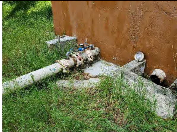
Figure 4. Outlet pipe to clearwell (center) and discharge to creek (right)
