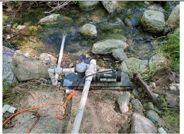
Figure 4. Temporary pumping system
