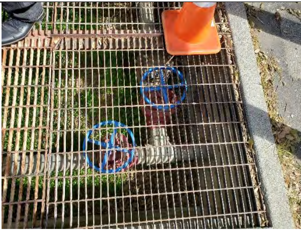
Figure 3. Water control valves
