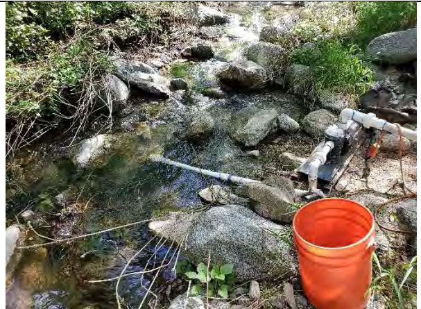
Figure 2. Temporary pumping system
