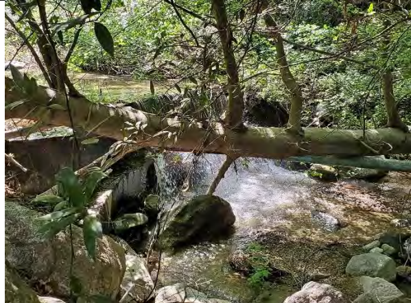
Figure 2. Fallen tree on 4-inch pipe near concrete box structure
