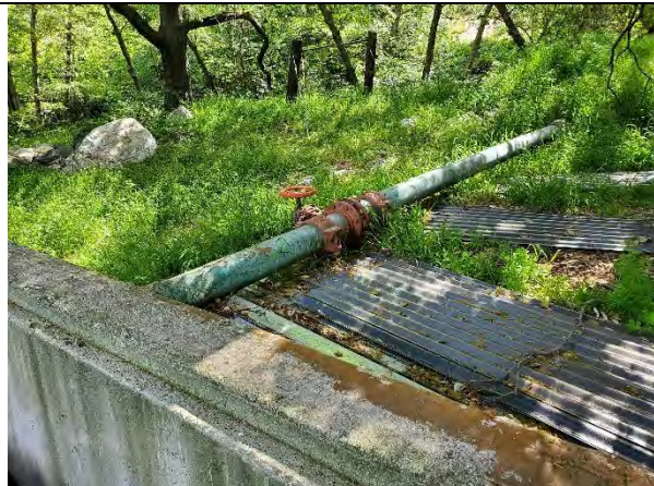
Figure 4. Steel pipe leading to sand filter
