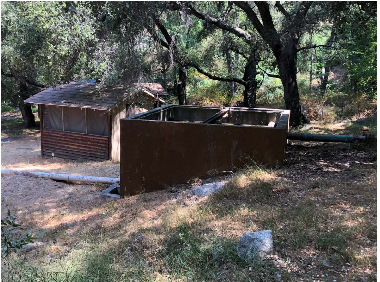
Photo 10: Existing slow sand filtration system
