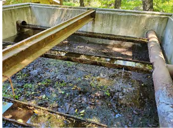
Figure 2. Pipes and conduits in filtration are rusted
