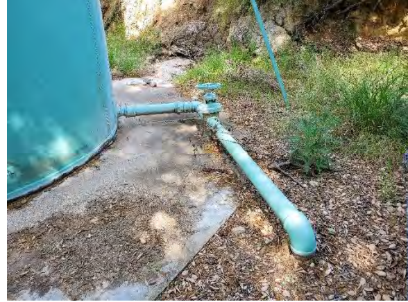
Figure 2. Inlet/outlet pipe for storage tank
