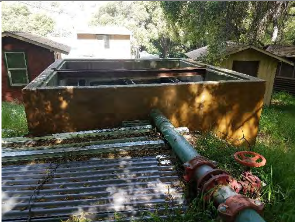
Figure 3. Inlet pipe going into the slow sand filter
