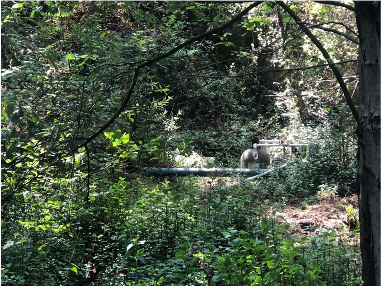
Photo 9: Sawpit wash pump station
