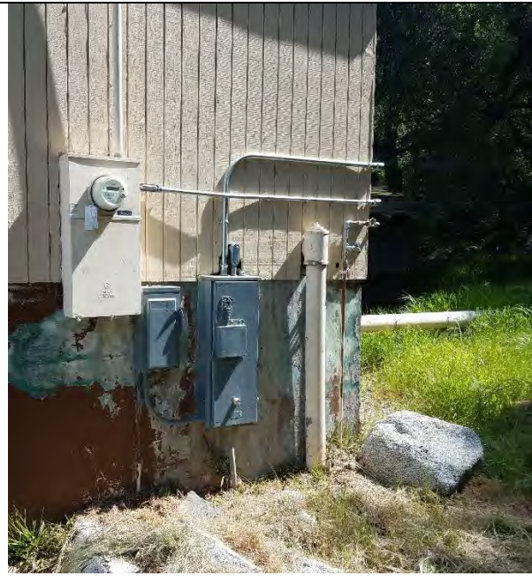
Figure 2. Electrical equipment on exterior of clearwell / pump house
