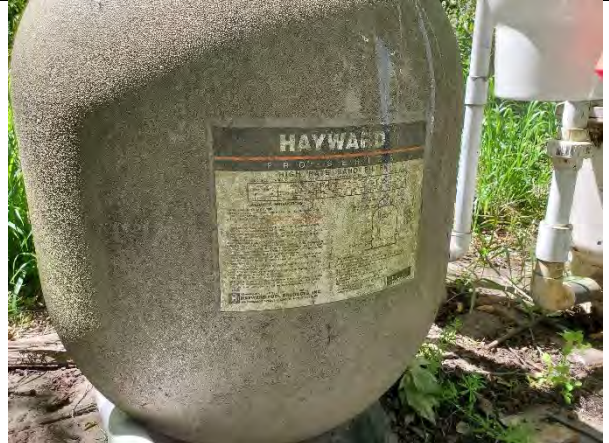
Figure 2. Rapid sand filter from pretreatment system
