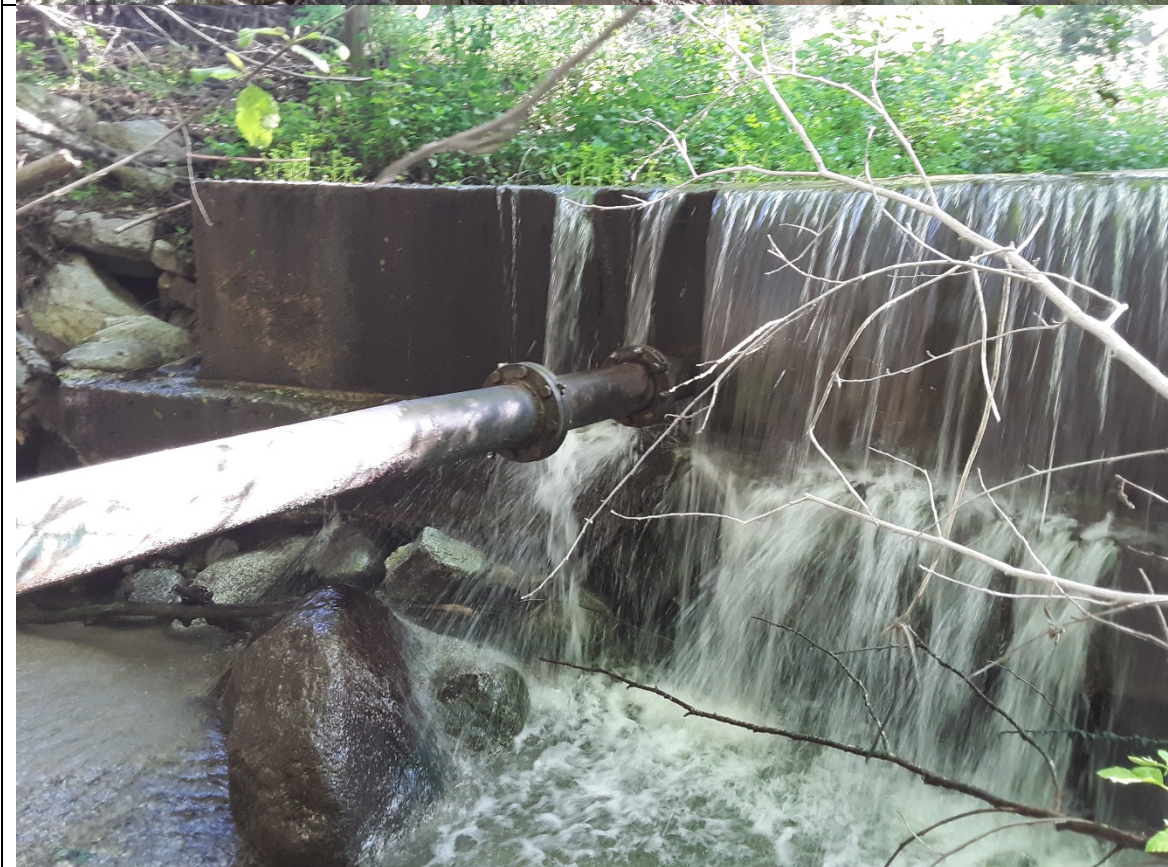
Photo 2. Intake pipe on downstream side of existing intake structure to remain in place.
