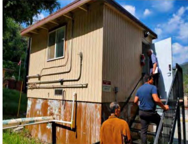
Photo 4: Clearwell / Pump House
