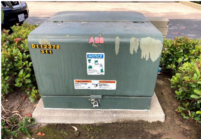
Photograph 3. View of the pad mounted transformer located on the southeastern boundary of the project site, facing southwest.
