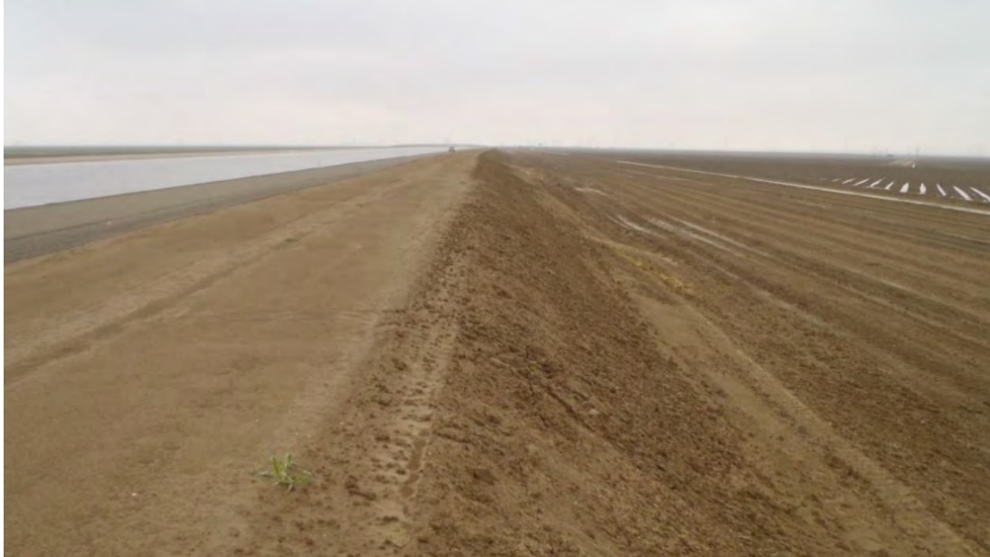
MP 135.23R - Raised embankment facing downstream next to agricultural land. Nearest occupied burrow location is MP 135.65R (January 14, 2017, Laura Castro).
