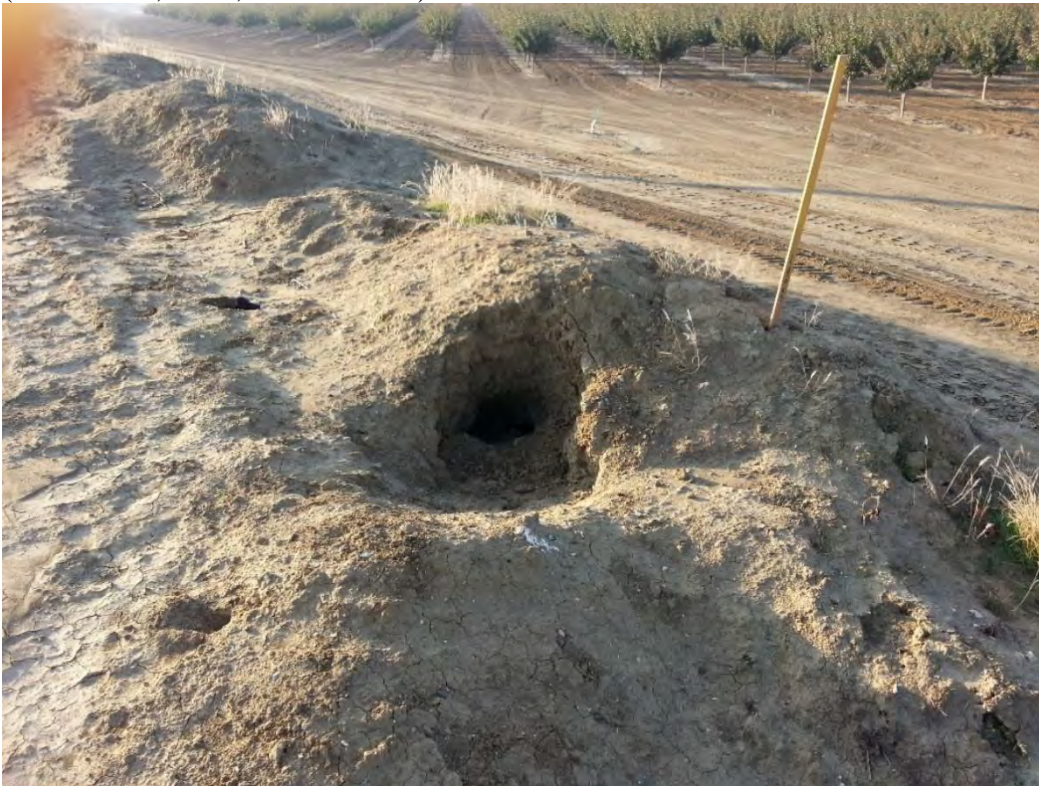
MP 140.05R - Occupied burrow with whitewash on top of embankment (October 17, 2016, Laura Castro).
