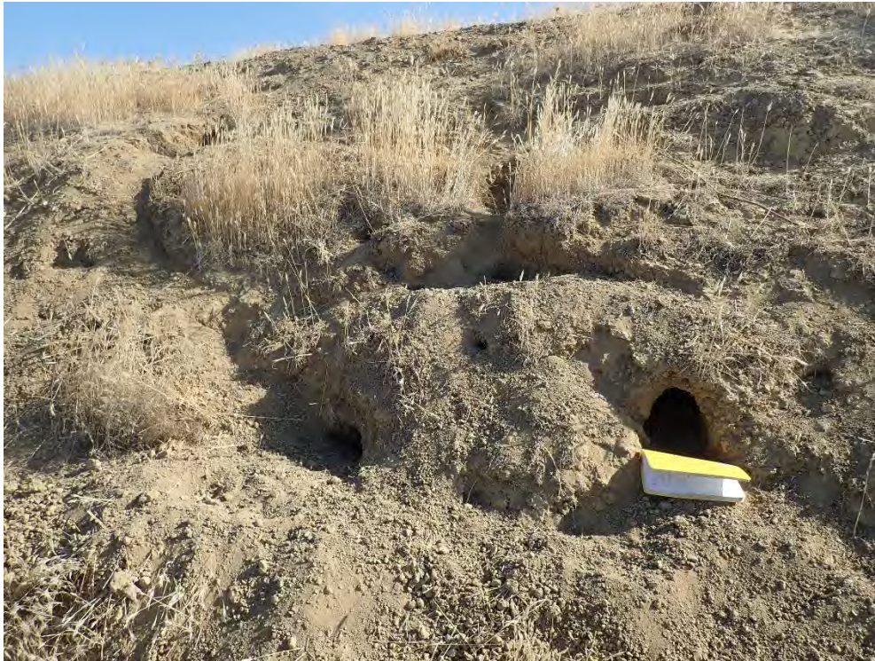
Figure 2. Small Mammal Burrow Complex near MP 140.50 Irrigation Crossing on the Right Side of the Aqueduct.
