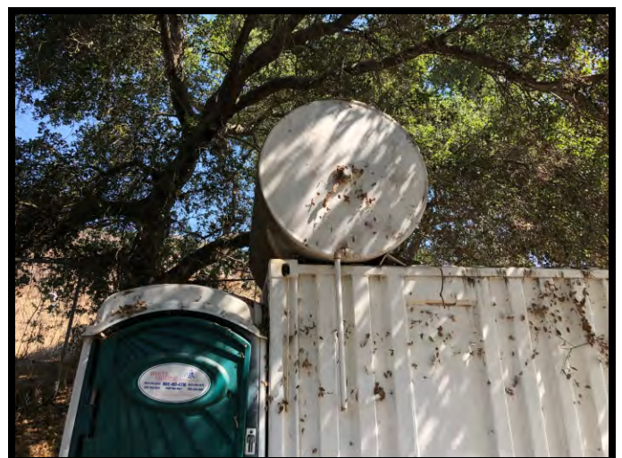
Photo #12: View of AST on top of container.
