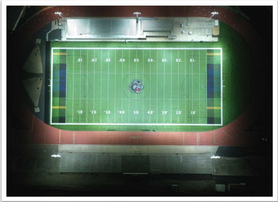
Figure 7, Similar Installed Examples of Proposed High-Mast Lighting System by Techline
