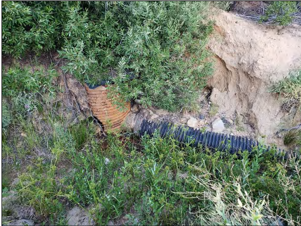
Photo 3. View of standpipe/culvert at the eastern terminus of the saturated section of the Intermittent Channel (CF4) (aspect southeast; 7/21/20).
