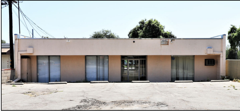
North (rear) elevation, view to the south (5/7/21). Note that parking lot is a few feet higher than the building entrance.
