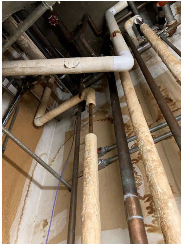
View of typical hardpack thermal system insulation considered an assumed ACM located in 150 N. Santa Anita Ave
