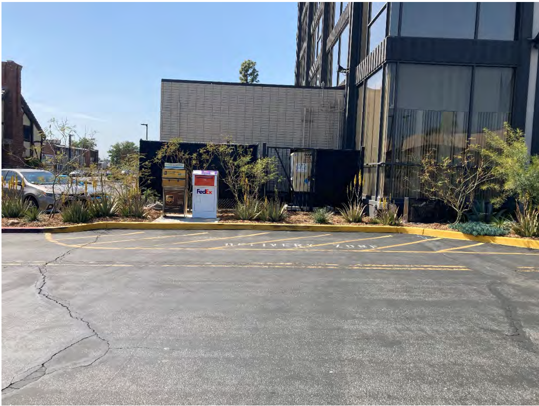
View of emergency backup generator compound containing two backup generators located on southeast side of the 150 N. Santa Anita Ave building
