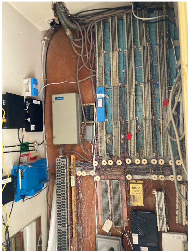
View of phone room at 25 Wheeler Ave
