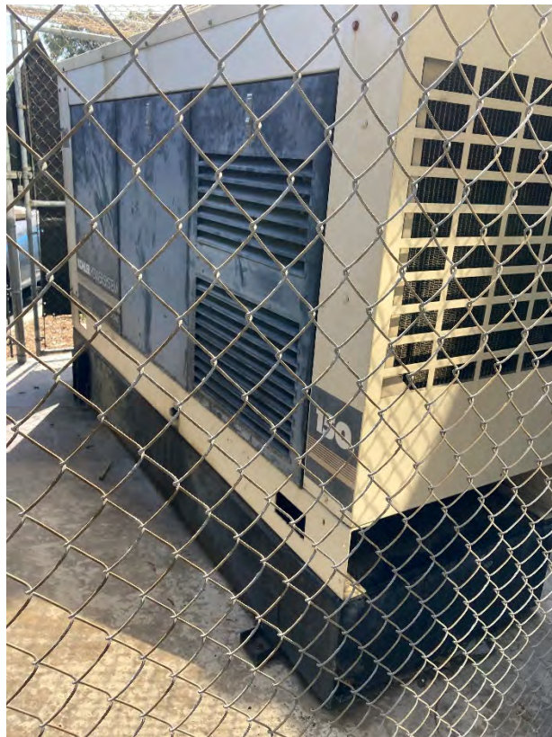
View of on-Site backup generator with base AST located on southeast side of 150 N. Santa Anita Ave building
