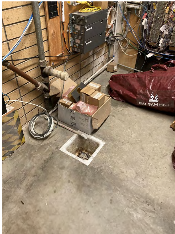
View of floor drain in equipment room/storage room of 150 N. Santa Anita Ave
