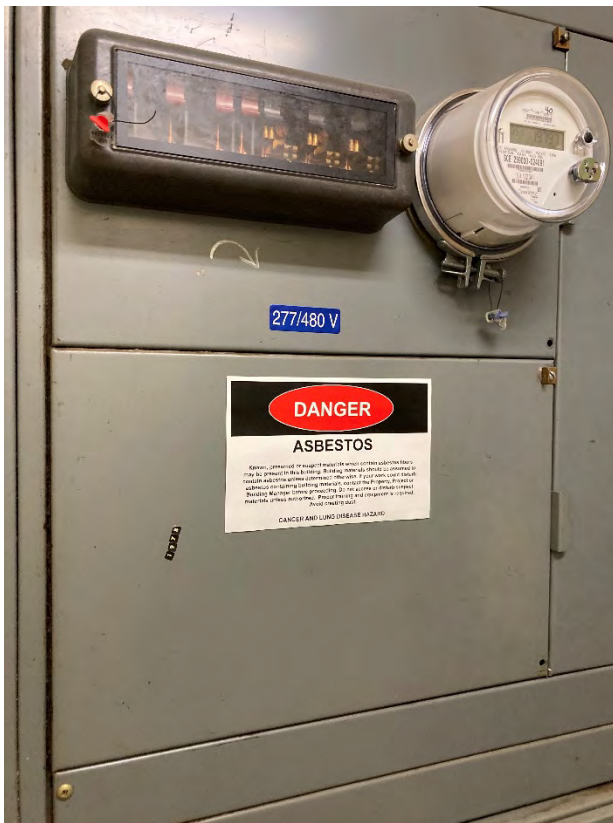
View of asbestos warning signs in 180 N. Santa Anita Ave
