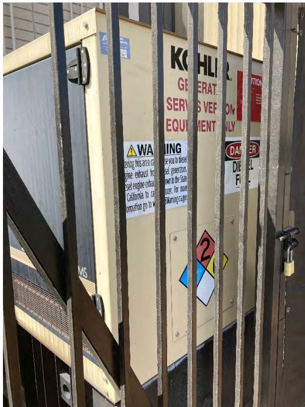
View of second backup generator with Diesel Fuel warning label located on southeast side of the 150 N. Santa Anita Ave building
