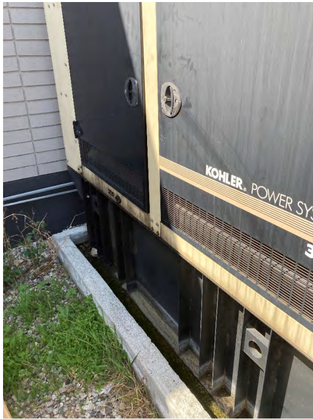
View of second backup generator with base AST located on southeast side of the 150 N. Santa Anita Ave building
