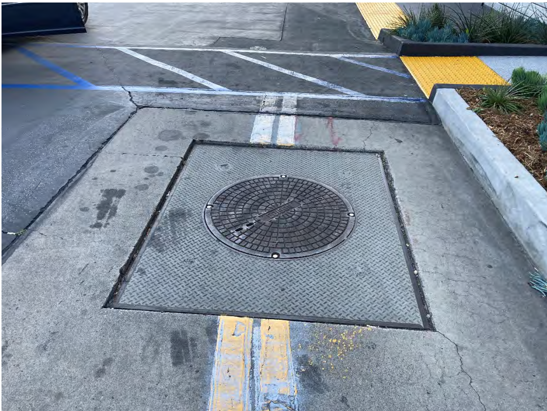
View of typical in-ground electrical access on Parcel B to east of the 150 N. Santa Anita Ave building
