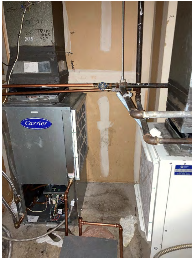
View of typical equipment located in equipment rooms on all floors of 150 N. Santa Anita Ave
