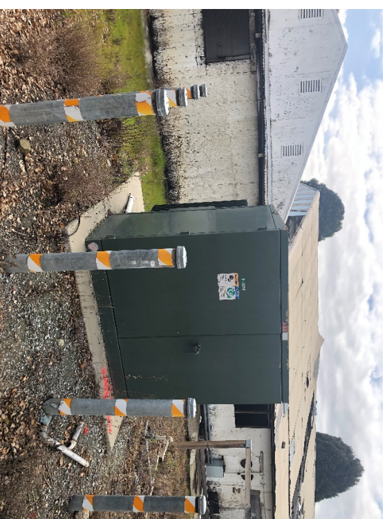
Photo 8: Transformer south of office building
