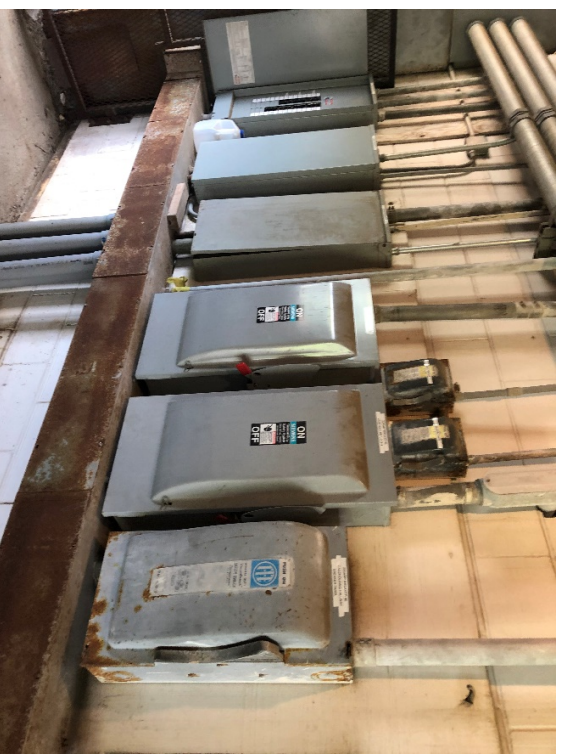
Photo 28: Western building electric panels
