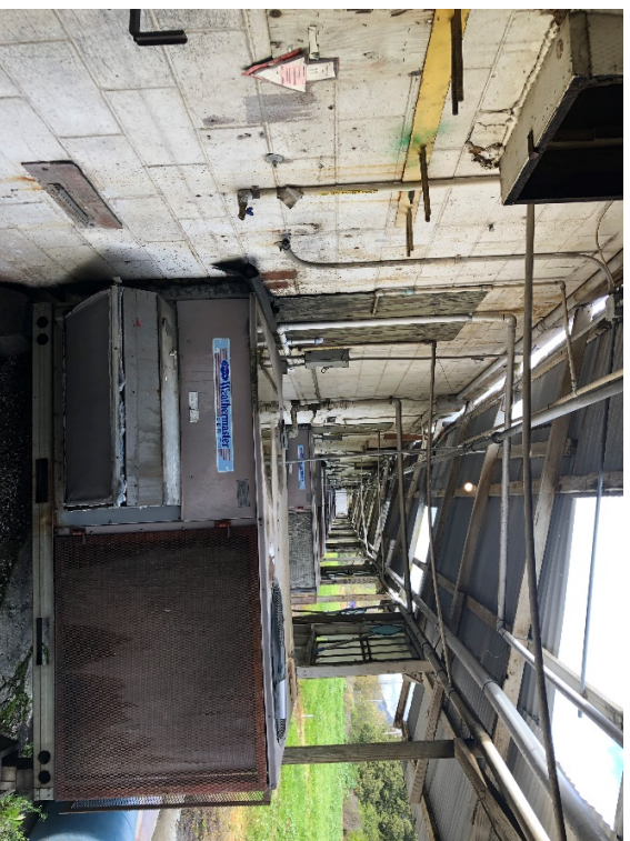
Photo 10: Heater units north end west drying buildings
